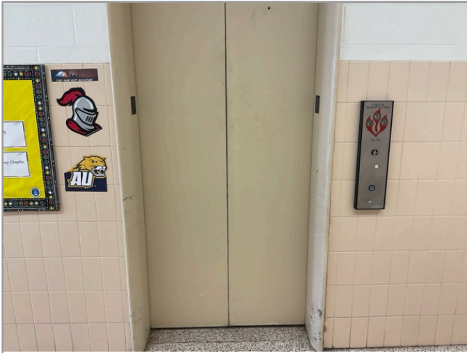
LOBBY LOOKING AT CAB
