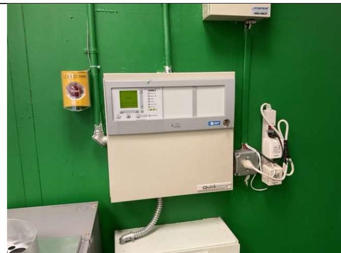
23 – FIRE ALARM PANEL
