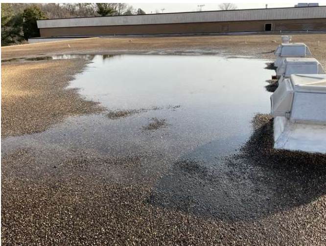
5 - STANDING WATER PRESENT ON ROOF
