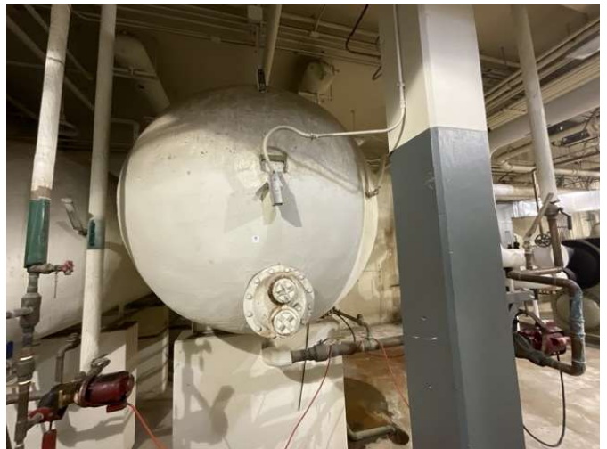
10 – DOMESTIC WATER STORAGE TANK
