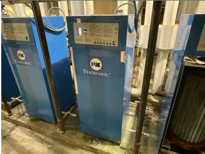
15 - MAIN MECHANICAL ROOM - HVAC BOILERS
