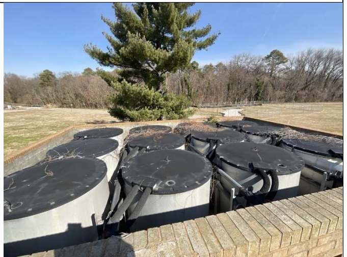
18 – ABANDONED HVAC THERMAL ICE STORAGE
