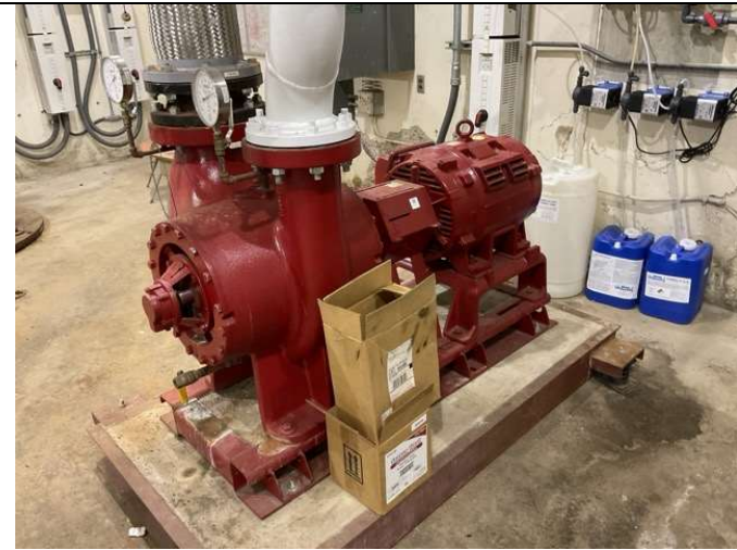
19 – HVAC DISTRIBUTION PUMP
