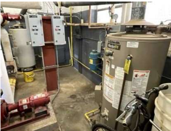
9 – DOMESTIC HOT WATER
