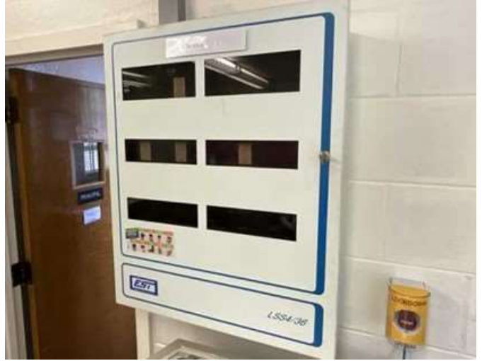
12 - FIRE ALARM CONTROL PANEL
