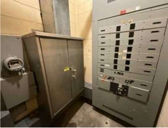
11 - MAIN ELECTRICAL ROOM
