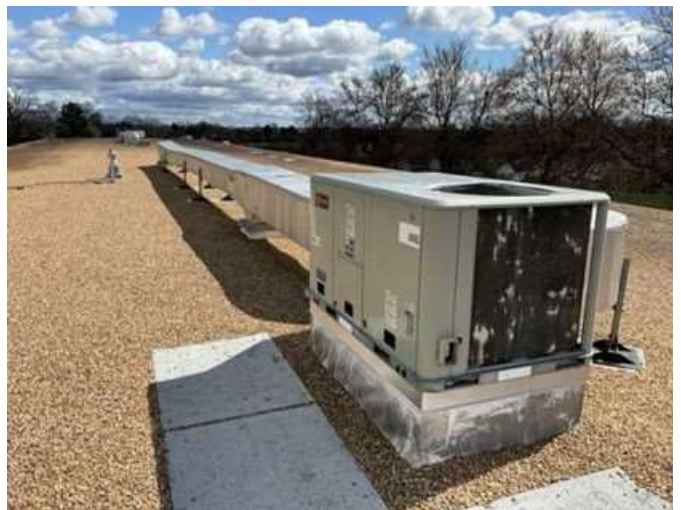
10 – ROOF MOUNTED PACKAGE UNIT
