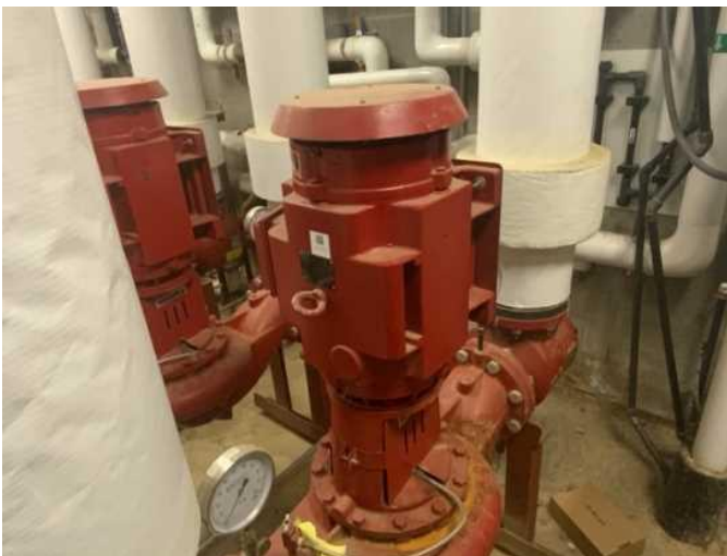
33 - HYDRONIC CIRCULATION PUMP
