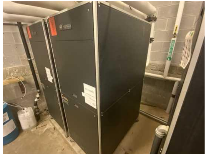
20 - WATER SOURCE HEAT PUMPS
