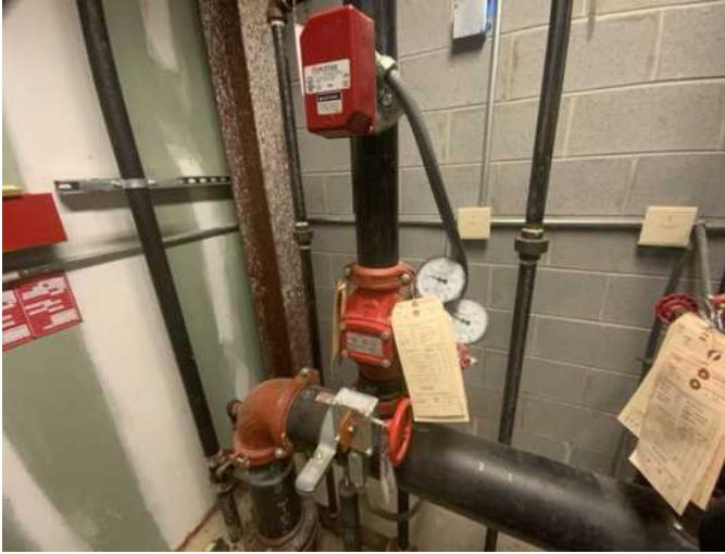
23 - FIRE SUPPRESSION SYSTEM
