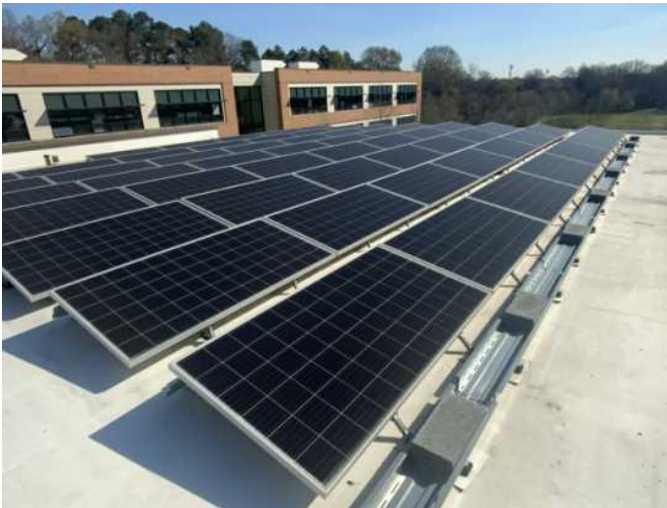
25 - SOLAR POWER PANELS
