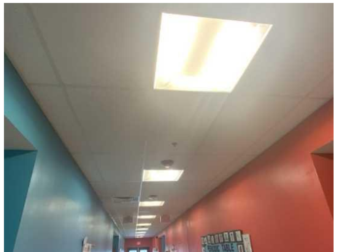
28 - INTERIOR LIGHTING SYSTEM
