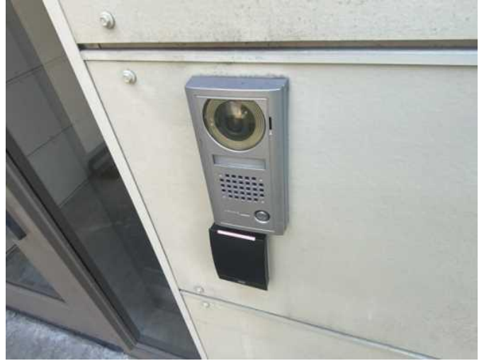
30 - INTRUSION DETECTION SYSTEM INTERCOM
