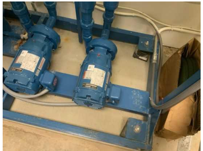
14 -DOMESTIC BOOSTER PUMP
