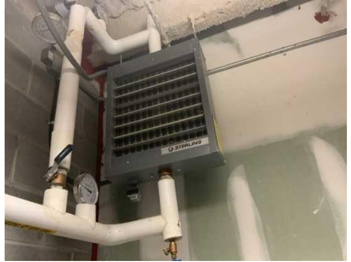
18 – HYDONIC UNIT HEATER
