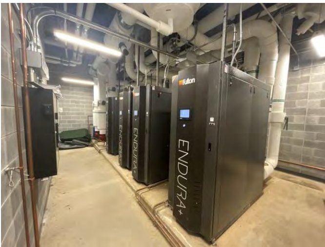
23 - MECHANICAL ROOM-HVAC BOILERS
