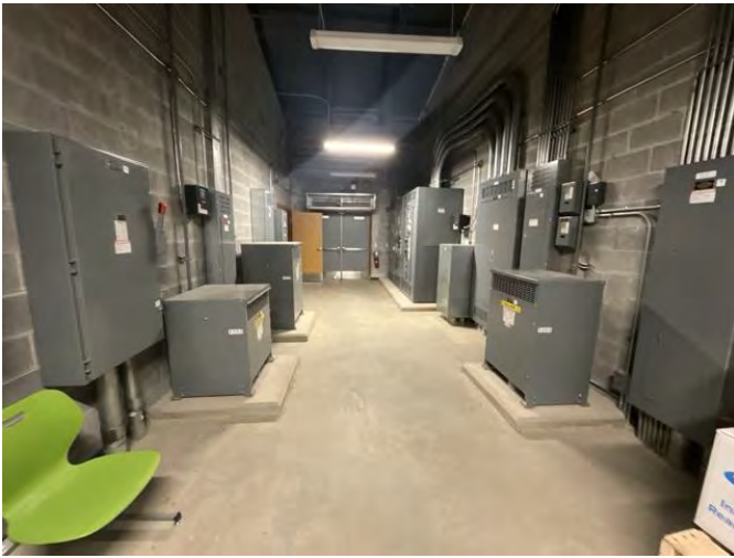
25 - MAIN ELECTRICAL ROOM
