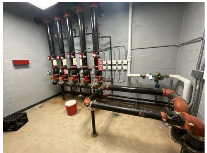
30 - FIRE RISER ROOM
