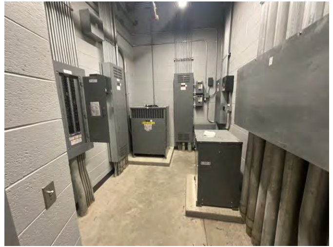
26 - SECONDARY ELECTRICAL ROOM
