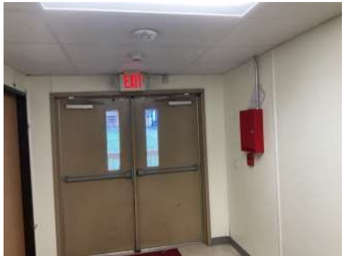
4 – FIRE ALARM SYSTEM
