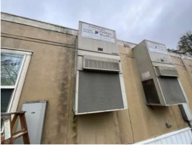
5 – WAKK-MOUNTED HEAT PUMPS
