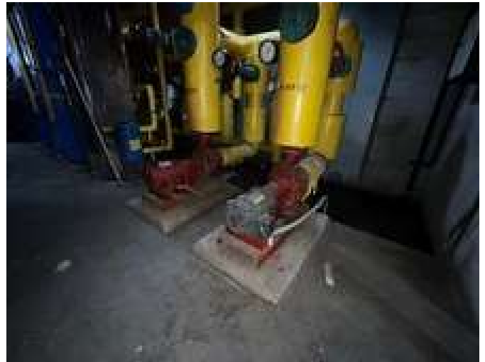
20 - BOILERS AND PUMPS
