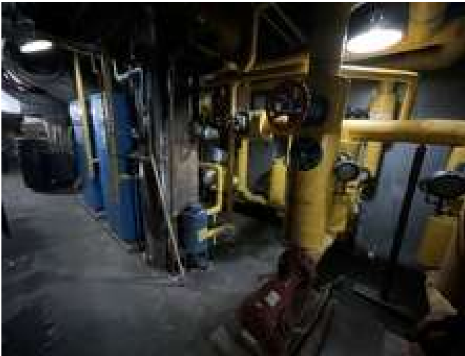
19 - MAIN MECHANICAL ROOM
