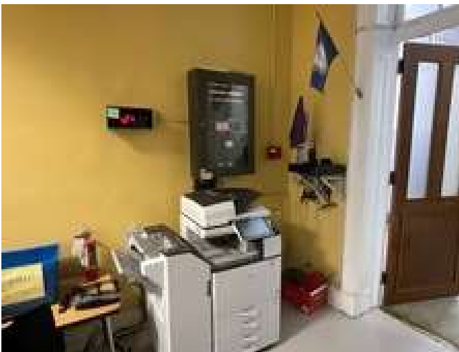
23 - FIRE ALARM PANEL
