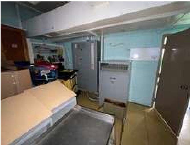
21 - MAIN ELECTRICAL ROOM
