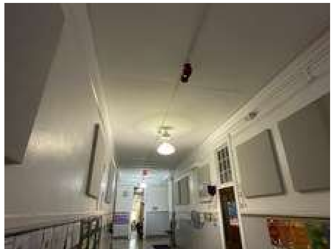
24 - FIRE EXTINGUISHER AND ALARM DEVICE
