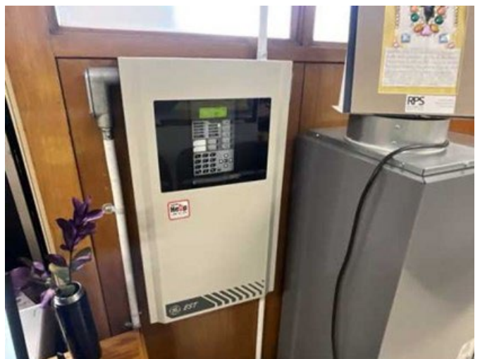
12 - FIRE ALARM CONTROL PANEL
