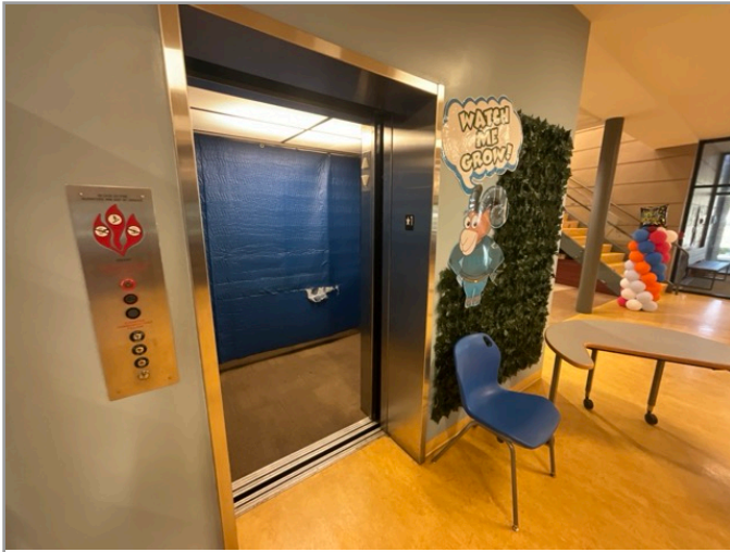
LOBBY LOOKING AT CAB
