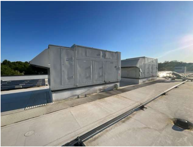
19 – ROOF TOP UNITS
