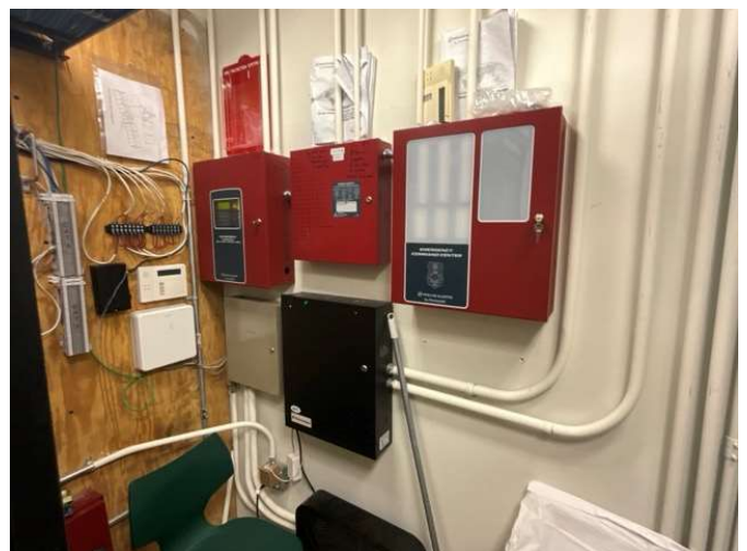
24 - FIRE ALARM PANEL
