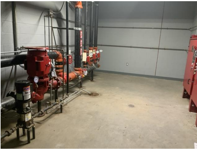
21 - FIRE SUPPRESSION SYSTEM
