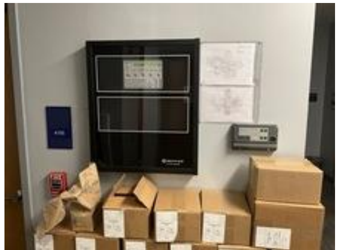
24 - FIRE ALARM PANEL
