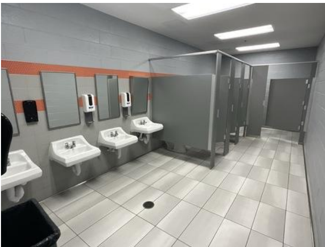
15 - DOMESTIC HOT WATER SUPPLY
