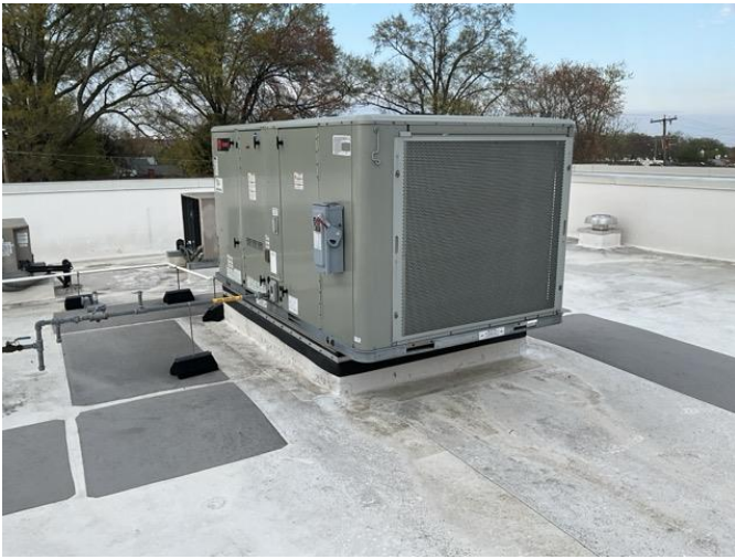
19 - ROOF TOP UNITS
