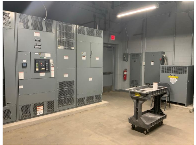
22 - MAIN ELECTRICAL SWITCHBOARD
