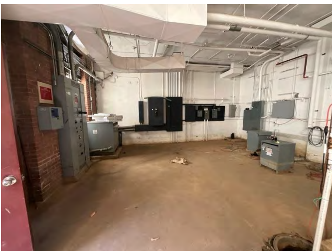
11 - MAIN ELECTRICAL EQUIPMENT
