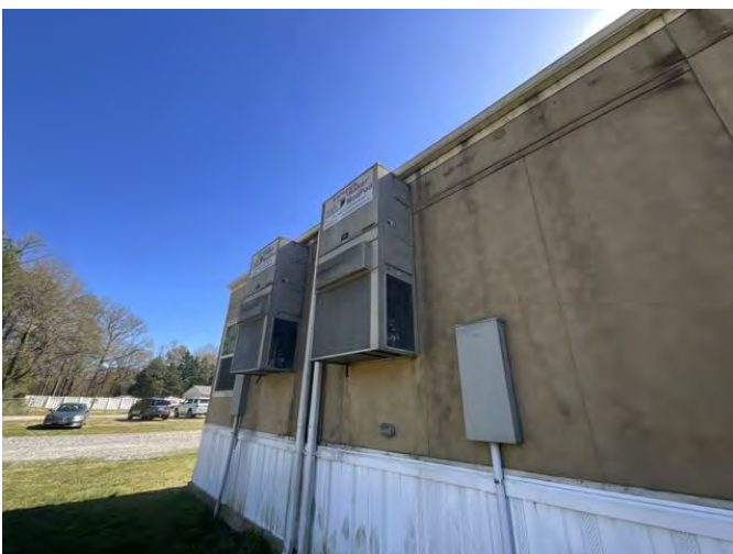
11 - WALL-MOUNTED HEAT PUMPS
