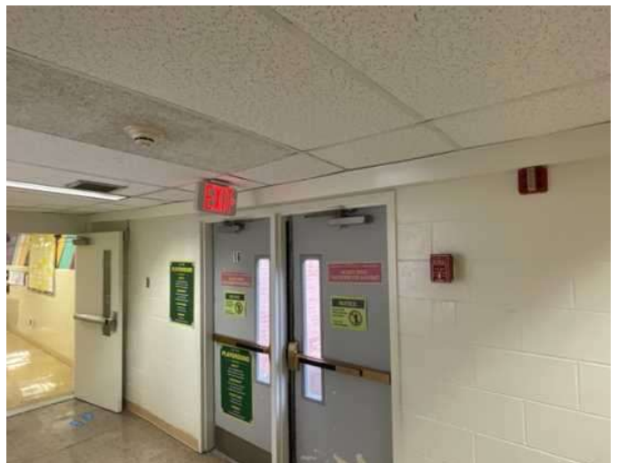
18 - FIRE ALARM SYSTEM COMPONENTS
