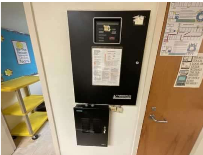
17 - FIRE ALARM PANEL
