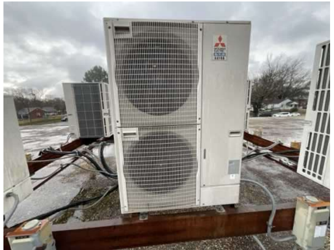
14 - ROOFTOP SPLIT SYSTEMS
