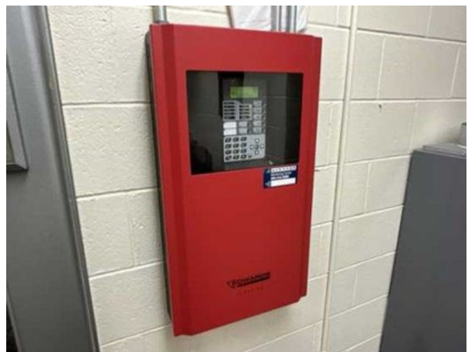
12 - FIRE ALARM CONTROL PANEL
