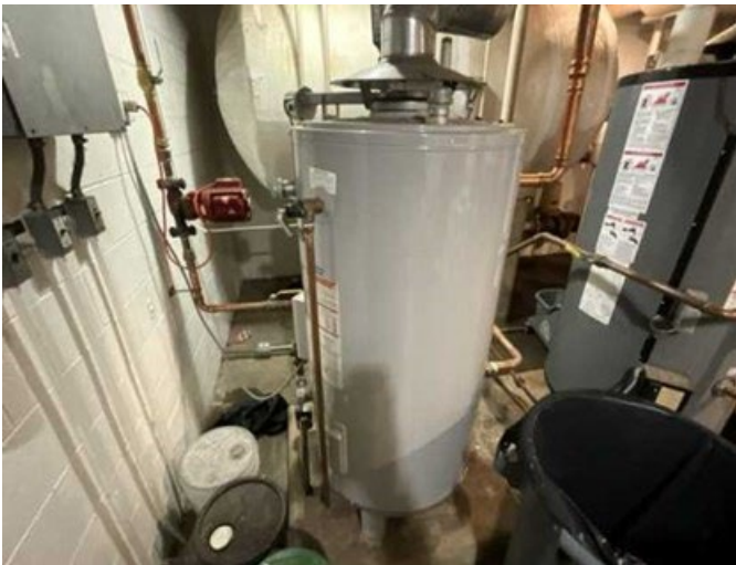
9 – DOMESTIC HOT WATER
