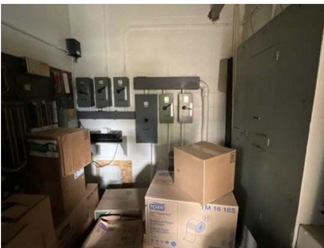
11 - MAIN ELECTRICAL ROOM
