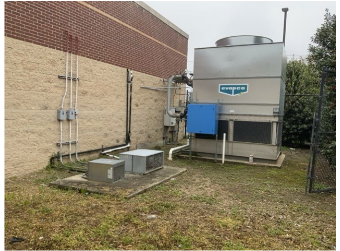
2 - COOLING TOWER ENCLOSURE
