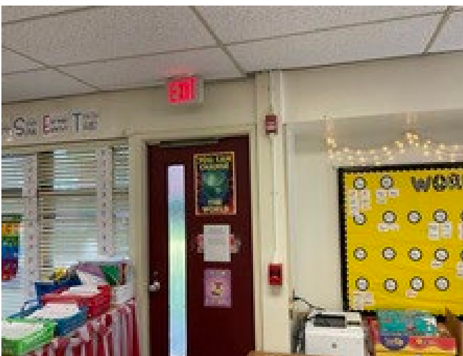
29 - FIRE ALARM DEVICES
