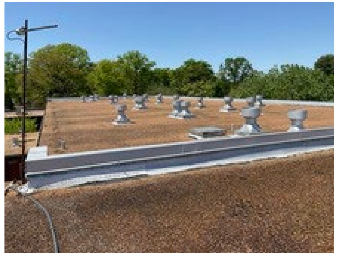
22 - ROOFTOP MECHANICAL EQUIPMENT
