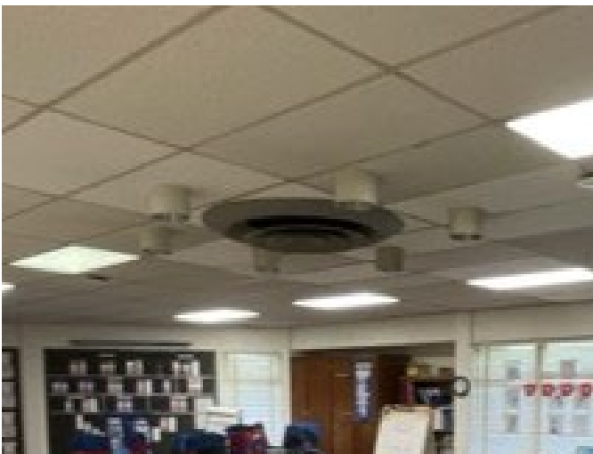
5 - HVAC SUPPLY DIFFUSER
