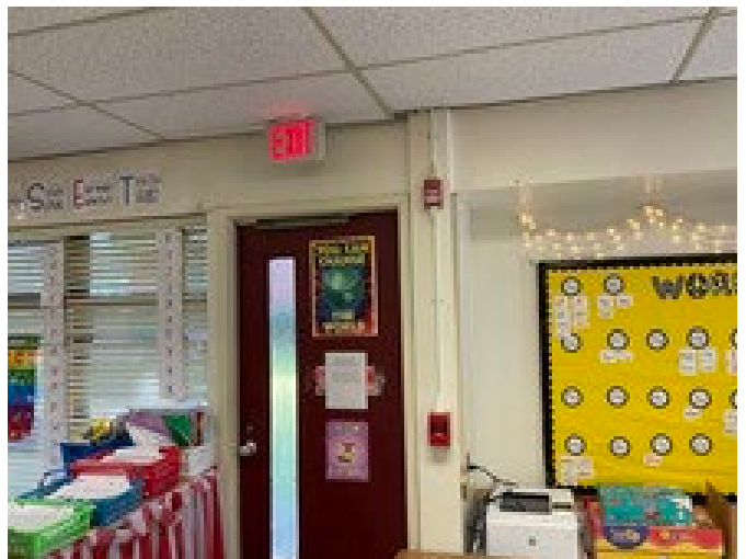
6 - FIRE ALARM DEVICES
