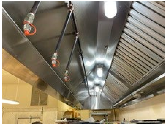
26 - FIRE SUPPRESSION SYSTEM
