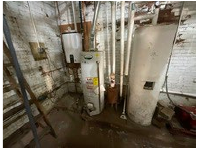
20 - DOMESTIC HOT WATER SUPPLY
