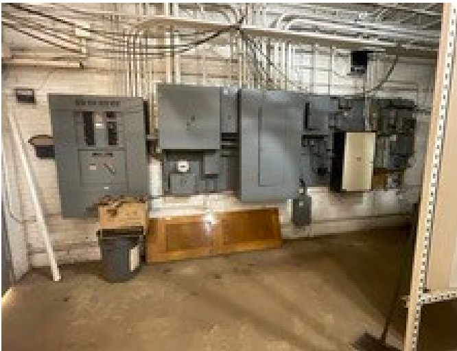
27 - MAIN ELECTRICAL ROOM
