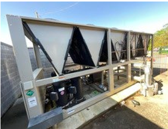
23 - CHILLERS AND PUMPS
