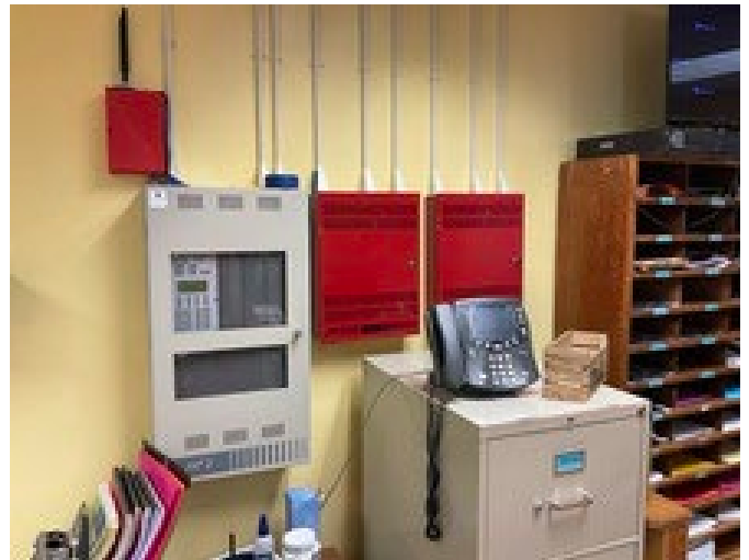
28 - FIRE ALARM SYSTEM
