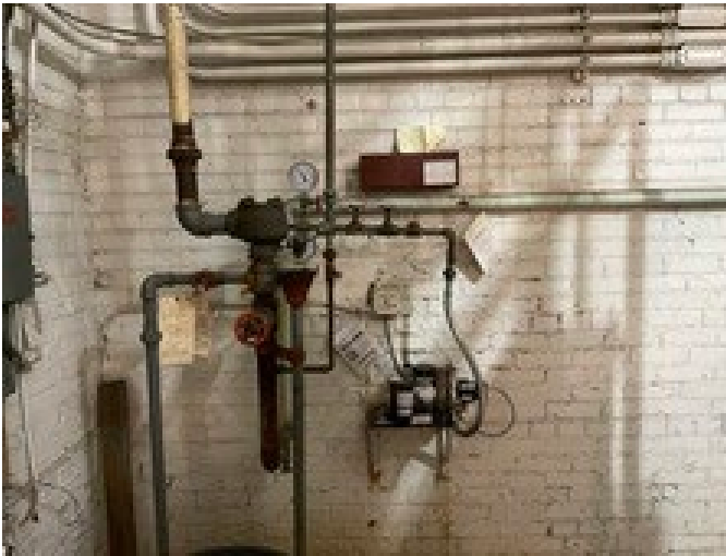
25 - FIRE SUPPRESSION SYSTEM
