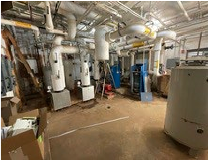
21 - MAIN MECHANICAL ROOM
