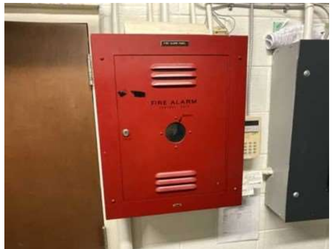
12 - FIRE ALARM CONTROL PANEL
