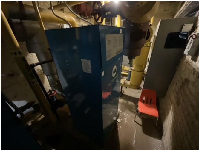
9 - MECHANICAL ROOM - HVAC BOILER
