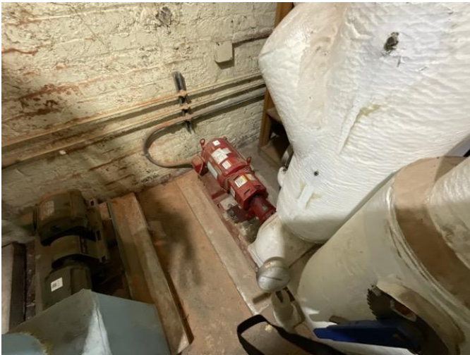
7 HEATING WATER DISTRIBUTION PUMP
