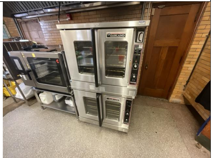
16 - COMMERCIAL KITCHEN EQUIPMENT
