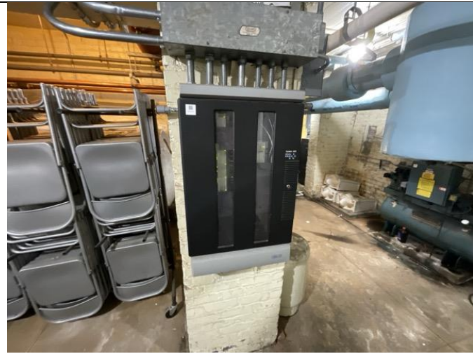
13 - BUILDING AUTOMATION SYSTEM CONTROLS
