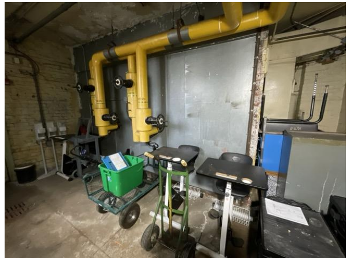
10 - MECHANICAL ROOM - AHU
