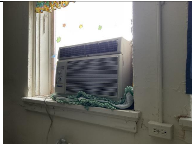
15 - WINDOW AC UNIT
