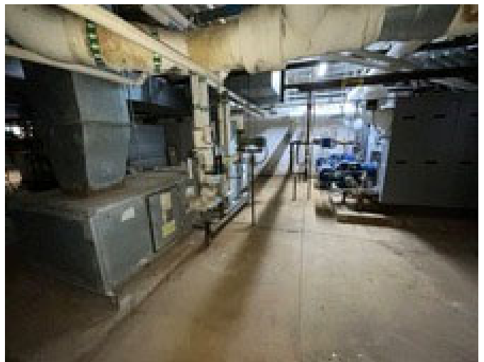
18 - MAIN MECHANICAL ROOM
