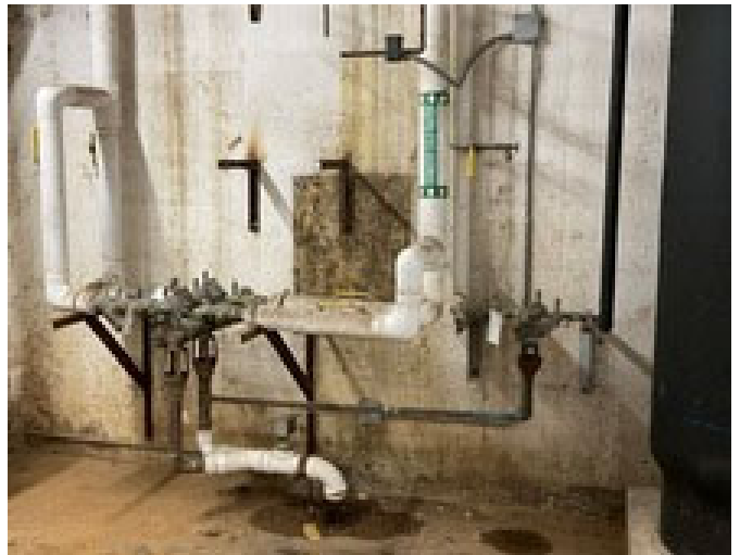
16 - DOMESTIC WATER PIPING
