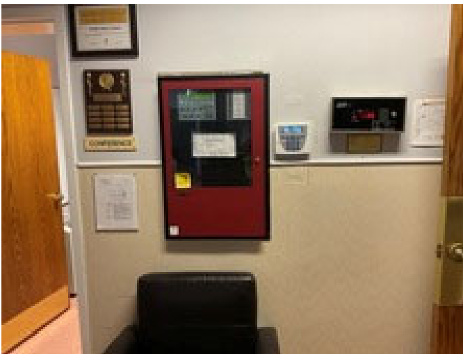
23 - FIRE ALARM PANEL
