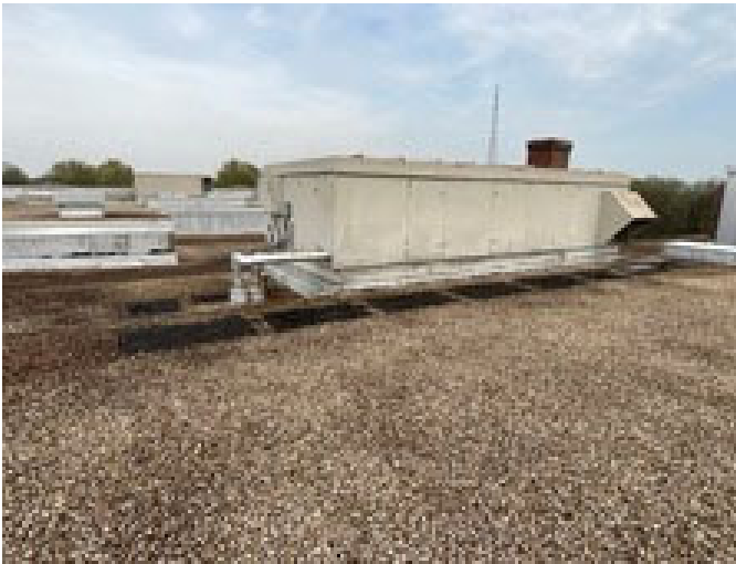
19 - ROOFTOP MECHANICAL EQUIPMENT
