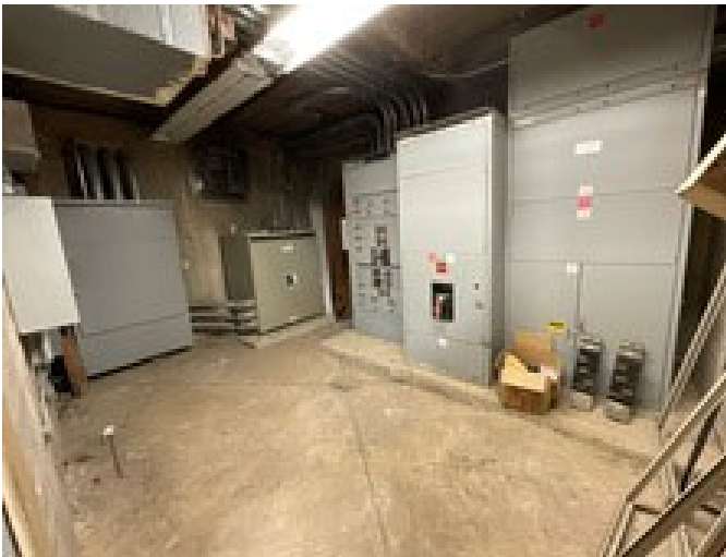
21 - MAIN ELECTRICAL ROOM
