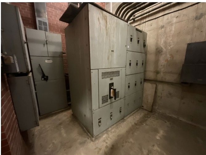
17 - MAIN ELECTRICAL SWITCHBOARD
