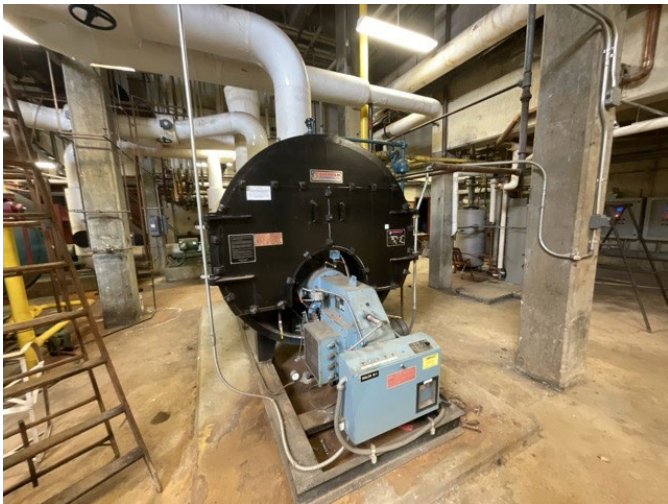
15 - MAIN MECHANICAL ROOM - HVAC BOILERS
