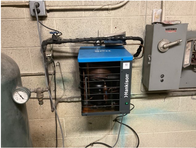
13 – COMPRESSED AIR DRYER
