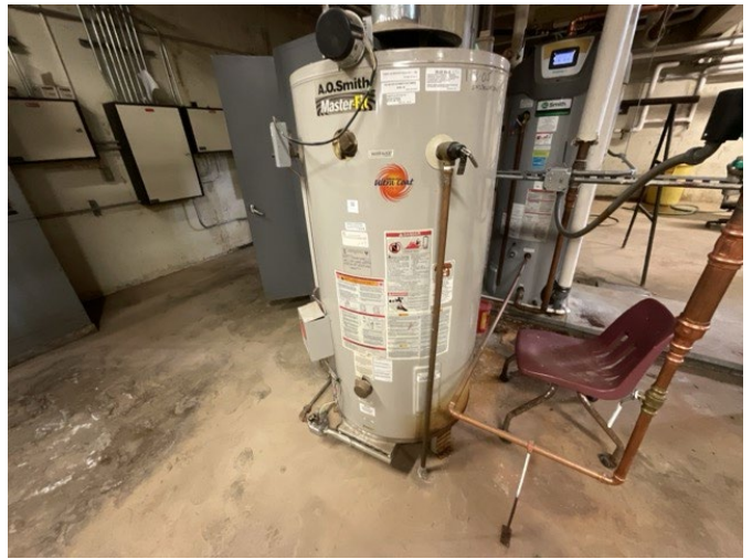
10 - GAS WATER HEATER
