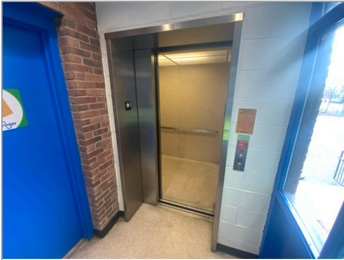
LOBBY LOOKING AT CAB
