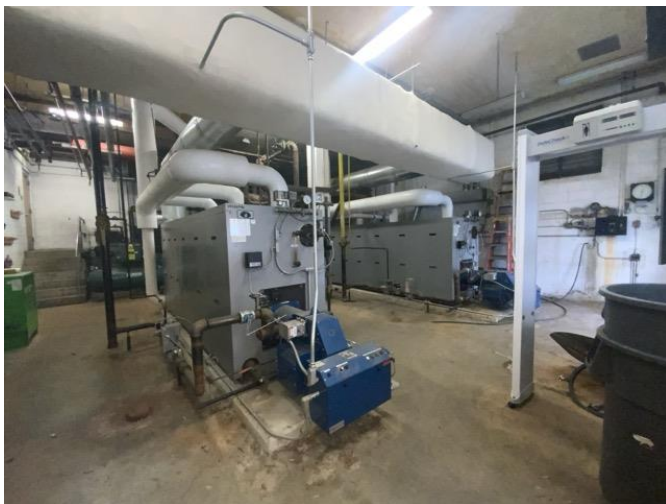
11 - MAIN MECHANICAL ROOM
