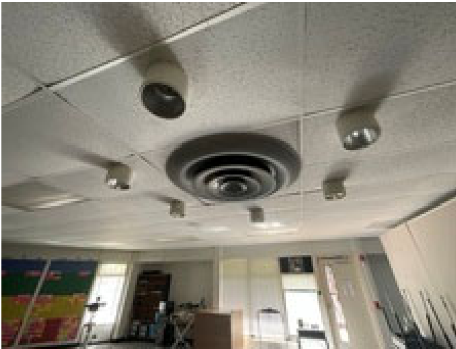
13 - CLASSROOM PACKAGED UNIT VENT
