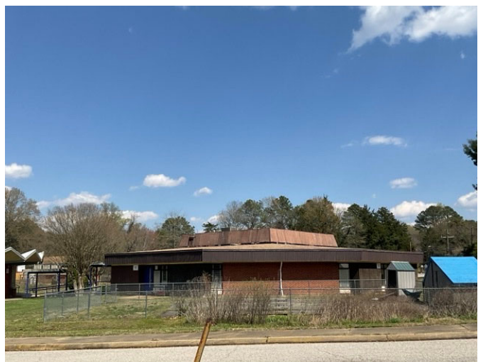
12 - PACKAGED UNITS ON ROOF
