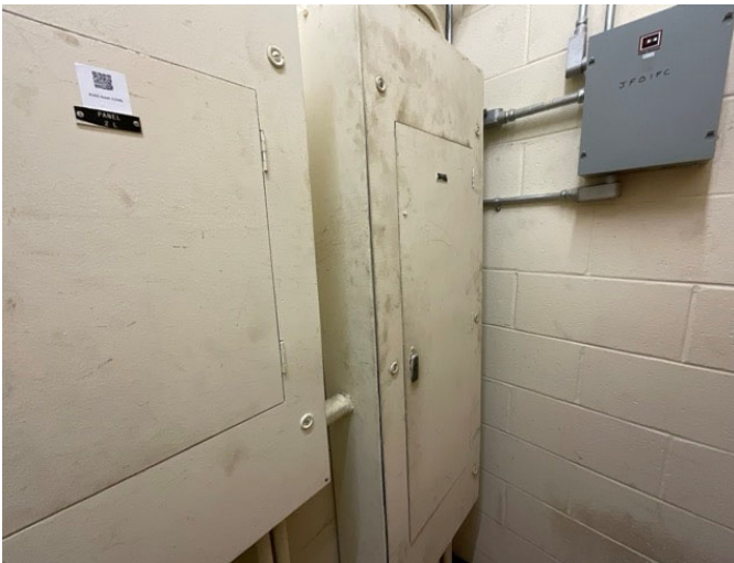
33 - FEDERAL PACIFIC ELECTRICAL PANELS
