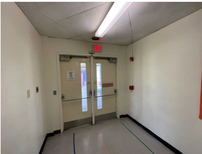
17 - FIRE ALARM DEVICES
