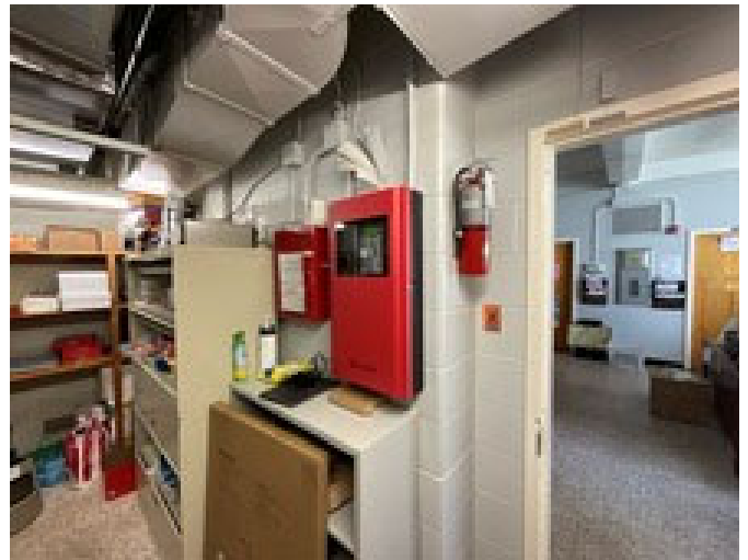
34 - FIRE ALARM CONTROL PANEL
