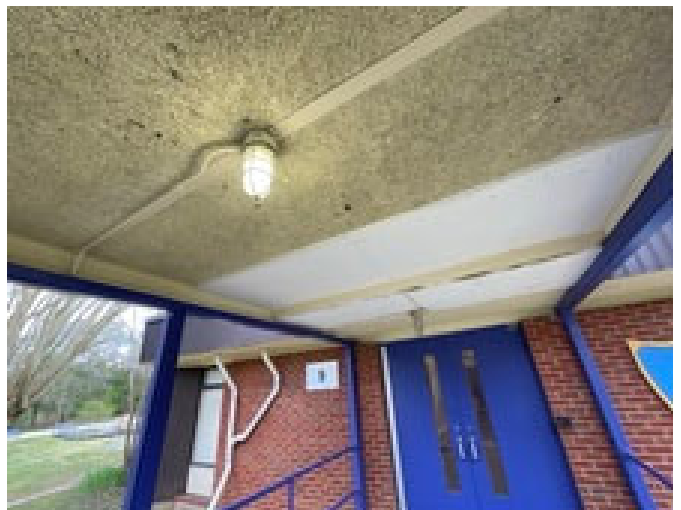
18 - BUILDING MOUNTED CFL FIXTURES
