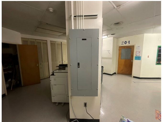
16 - SUPPLEMENTAL DISTRIBUTION PANEL
