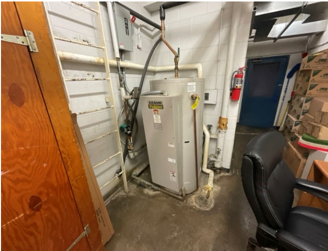
25 - LARGE ELECTRIC WATER HEATER
