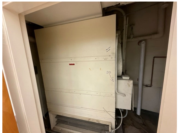
30 - INTERIOR AIR HANDLING UNIT
