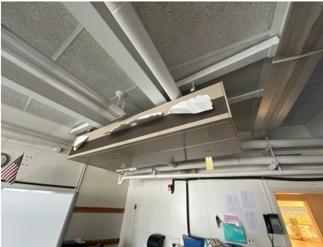
31 - CLASSROOM FAN COIL UNIT
