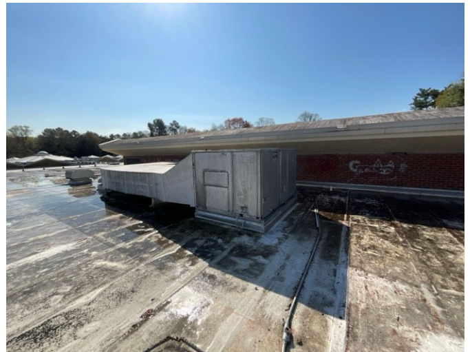
28 - ROOFTOP PACKAGED UNIT
