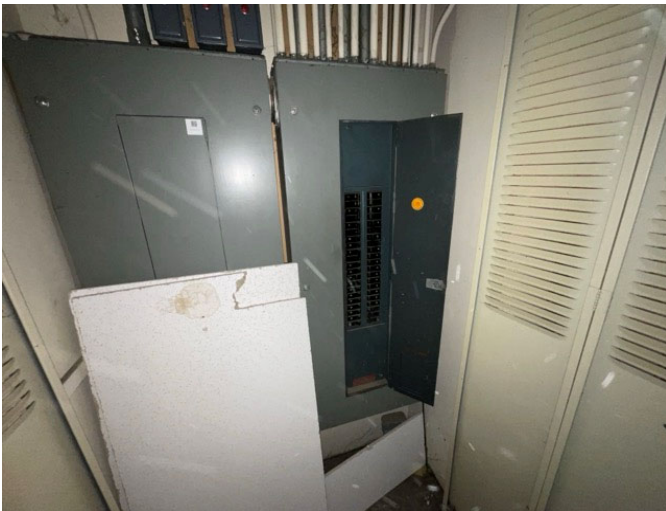
15 - MAIN ELECTRICAL EQUIPMENT
