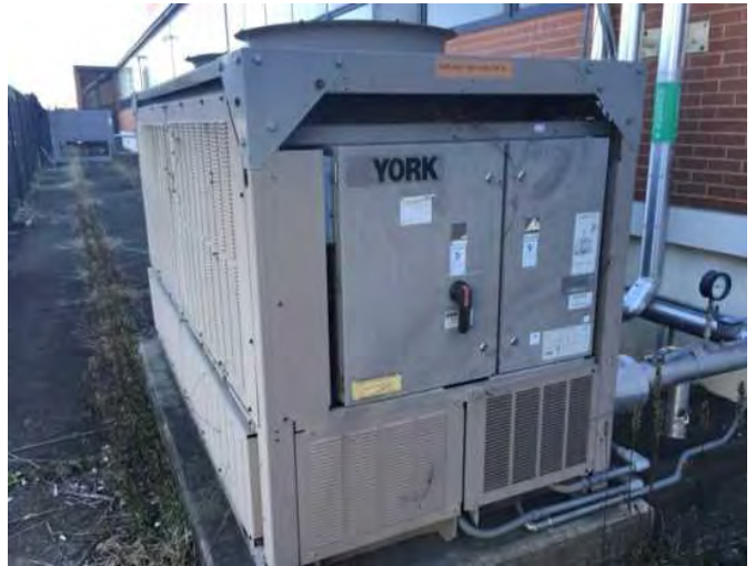
32 - AIR COOLED CHILLER
