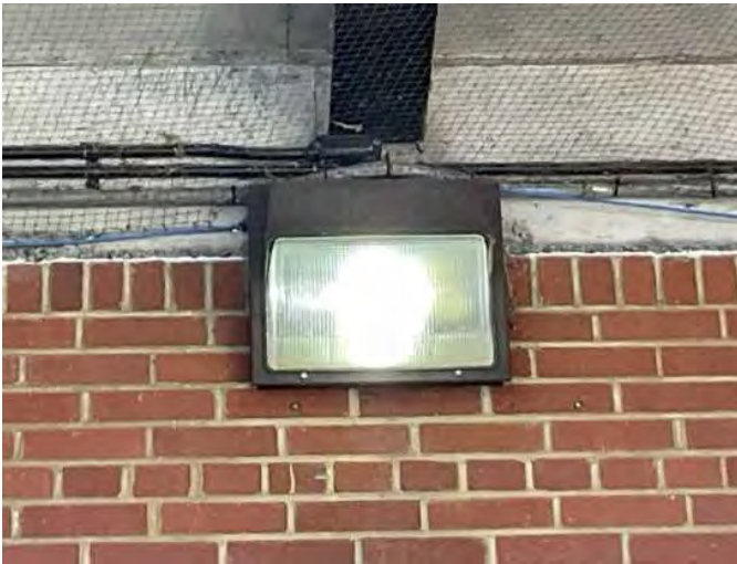
7 - EXTERIOR SITE LIGHTING
