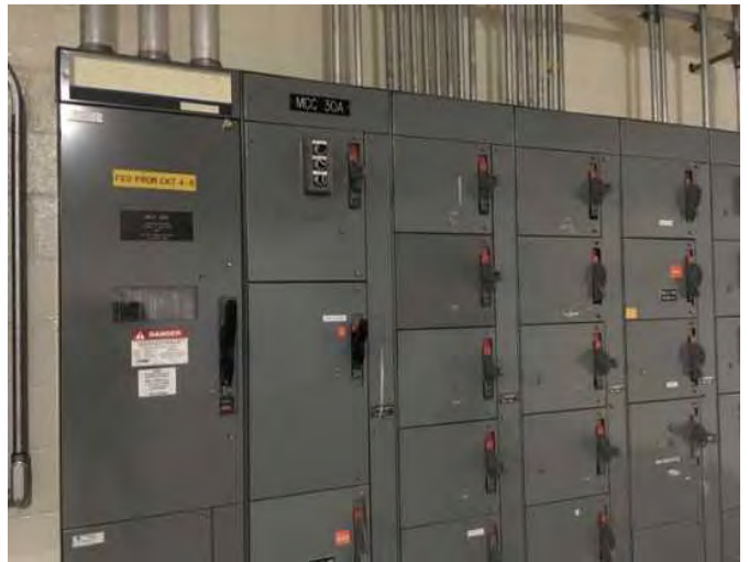
34 - MOTOR CONTROL CENTER
