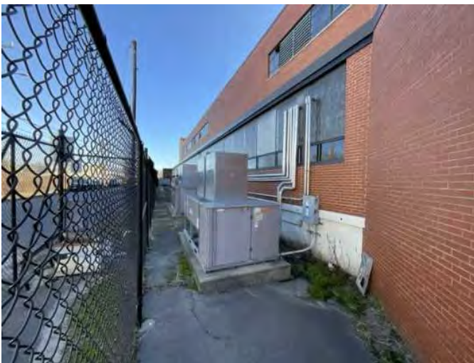
17 - BUILDING EXTERIOR CONDENSING UNITS
