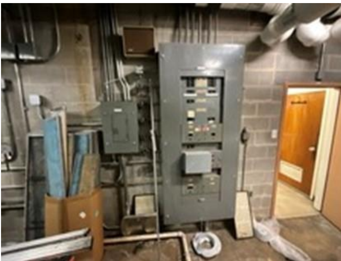
11 - MAIN ELECTRICAL ROOM
