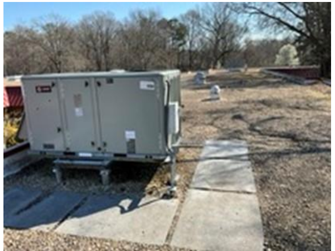
10 - ROOF MOUNTED PACKAGE UNIT
