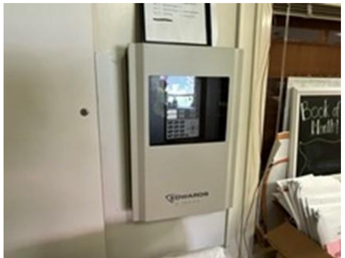
12 - FIRE ALARM CONTROL PANEL
