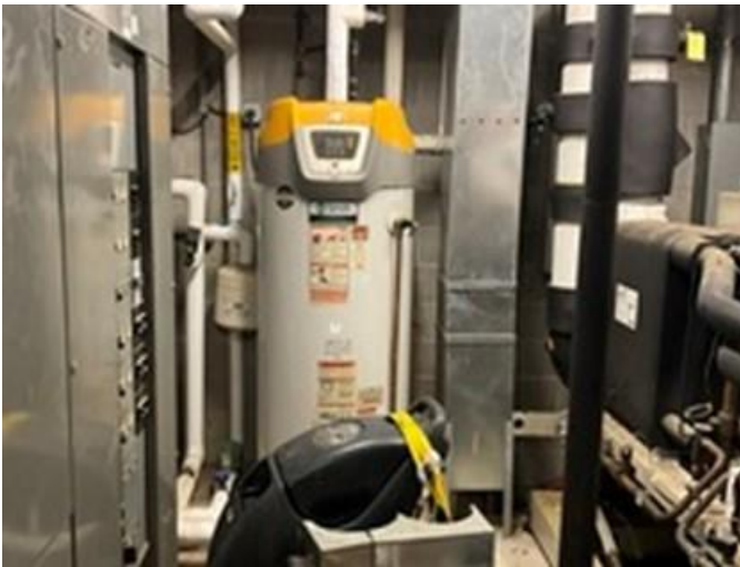
9 - DOMESTIC HOT WATER
