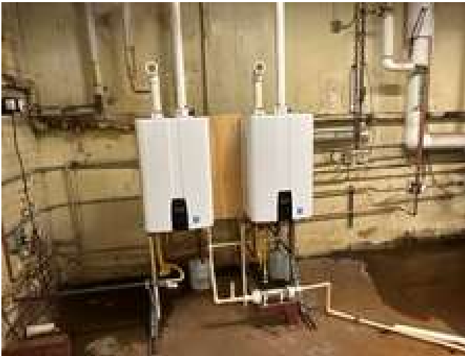
13 - DOMESTIC HOT WATER SUPPLY
