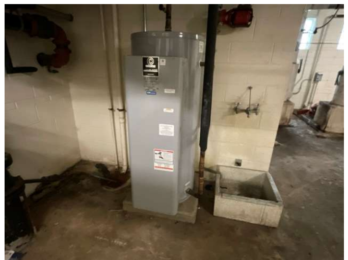
12 - DOMESTIC HOT WATER SUPPLY
