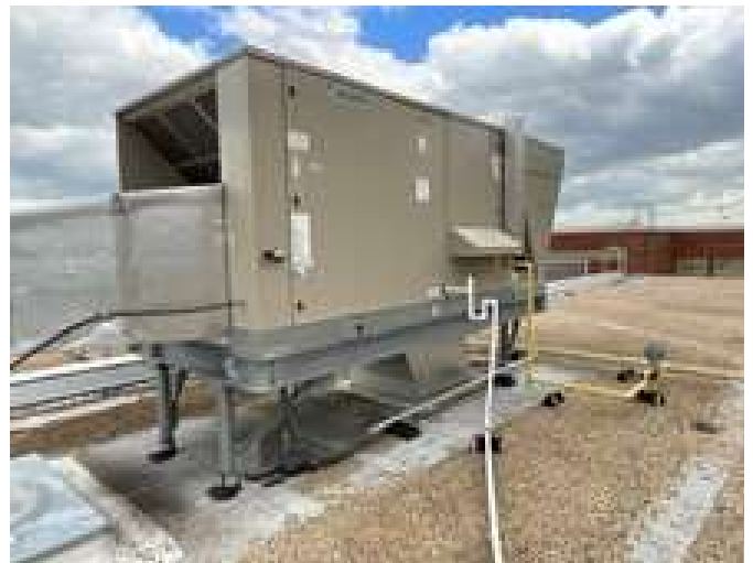
16 - ROOFTOP MECHANICAL EQUIPMENT
