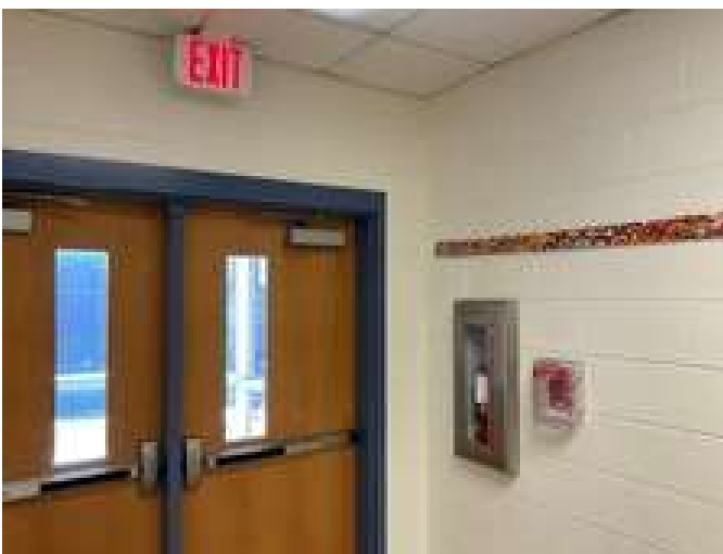
23 - FIRE EXTINGUISHERS AND ALARM DEVICES
