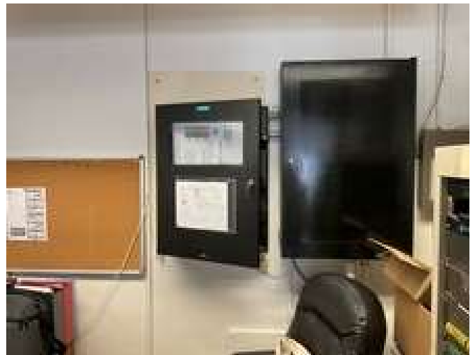
22 - FIRE ALARM PANEL
