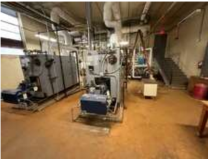
15 - MAIN MECHANICAL ROOM
