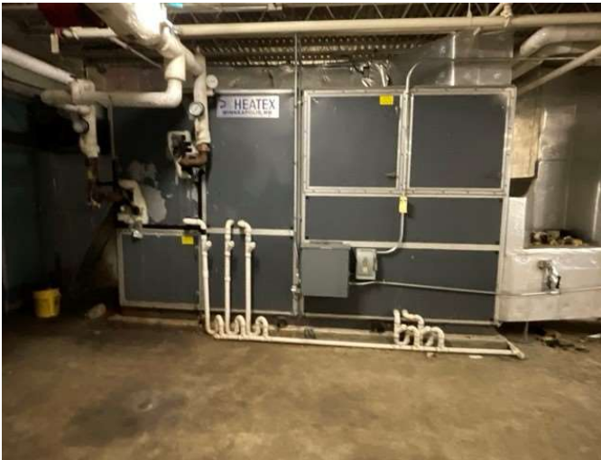
13 - AIR HANDLING UNIT
