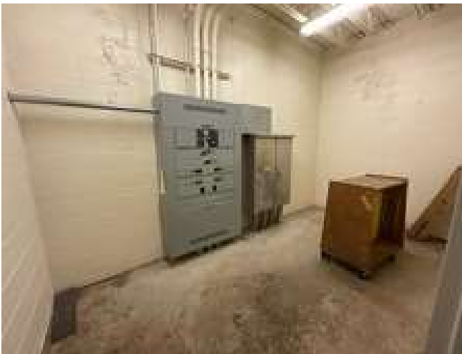
21 - MAIN ELECTRICAL ROOM
