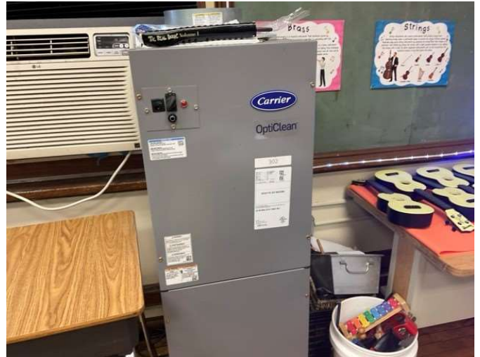
10 - CLASSROOM AIR PURIFIER
