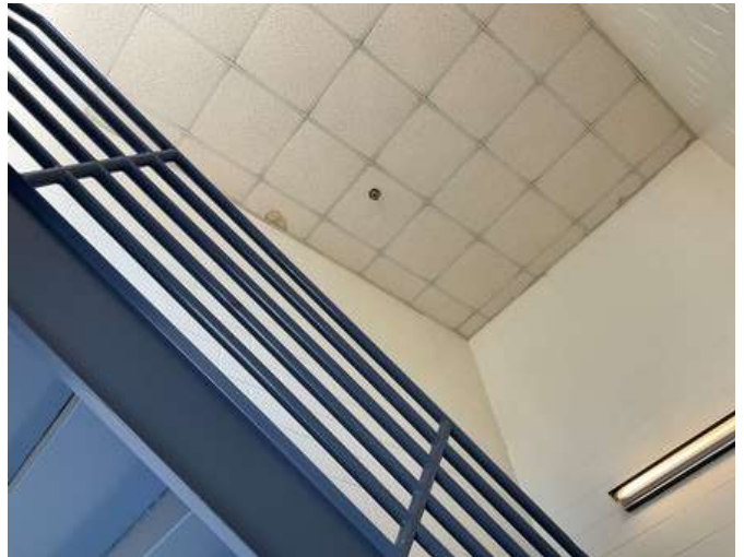
20 - STAIRWELL SPRINKLER HEAD
