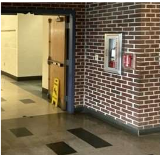
23 - FIRE EXTINGUISHER AND ALARM DEVICES
