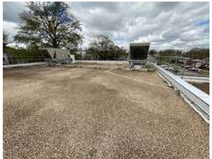
16 - ROOFTOP MECHANICAL EQUIPMENT
