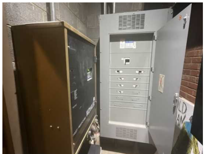
22 - Main Electrical Panel
