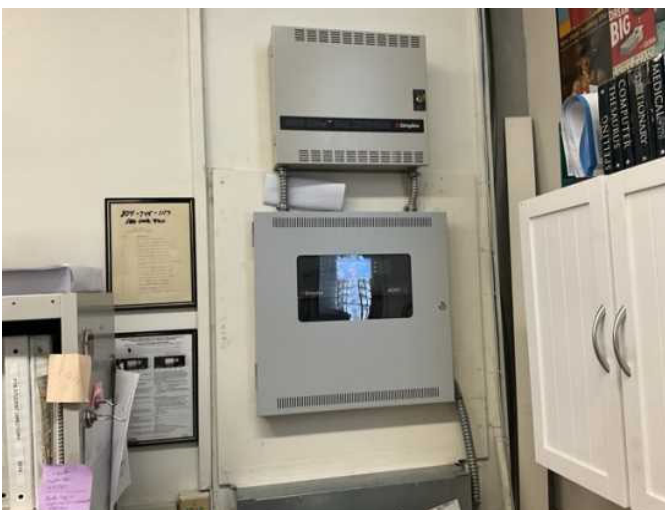
21 - Fire Alarm Panel
