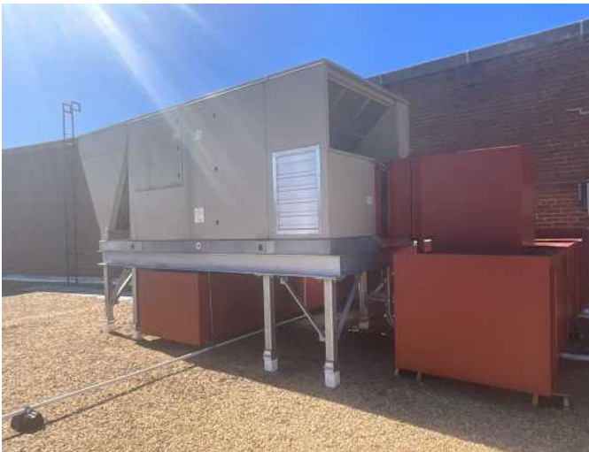
19 - HVAC, Rooftop Unit
