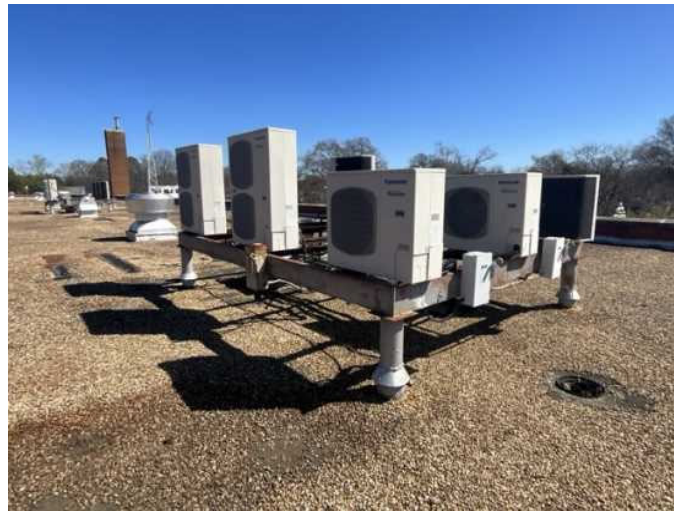
20 - HVAC, Split system units
