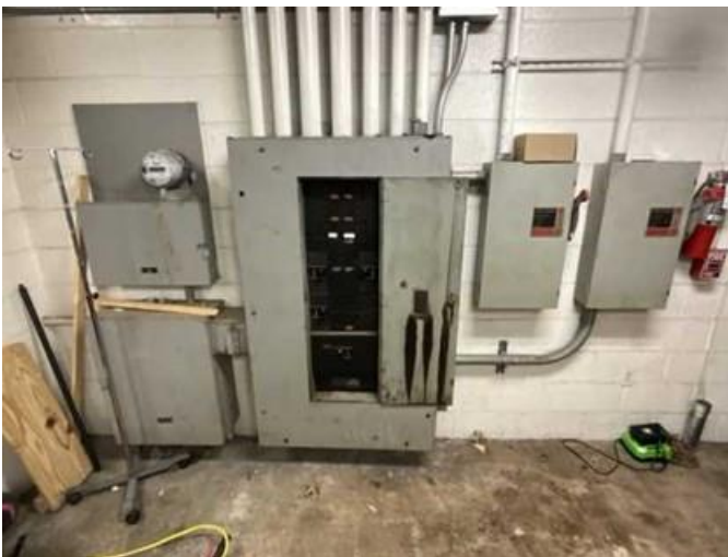
11 - MAIN ELECTRICAL ROOM
