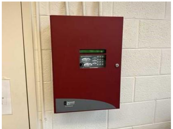
12 - FIRE ALARM CONTROL PANEL
