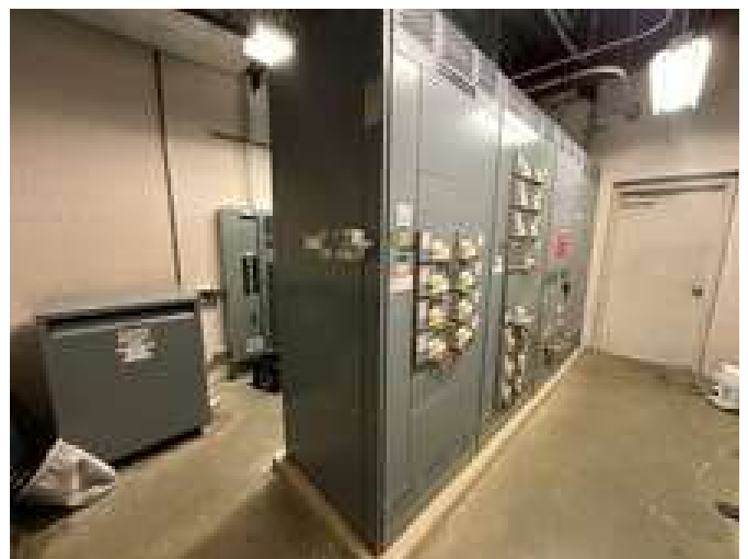
6 - PRIMARY ELECTRICAL ROOM
