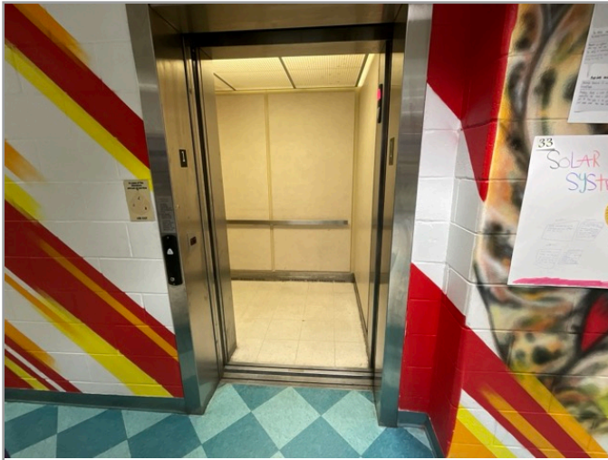
LOBBY LOOKING AT CABS (WITH DOORS OPEN)
