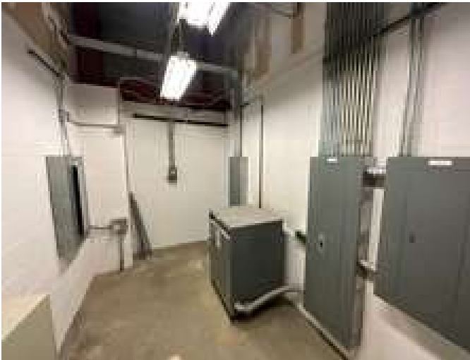
7 - SECONDARY ELECTRICAL ROOM
