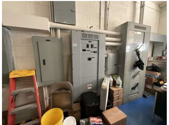
22 - Main Electrical Panel
