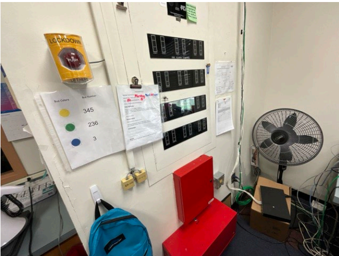
21 - Fire Alarm Panel
