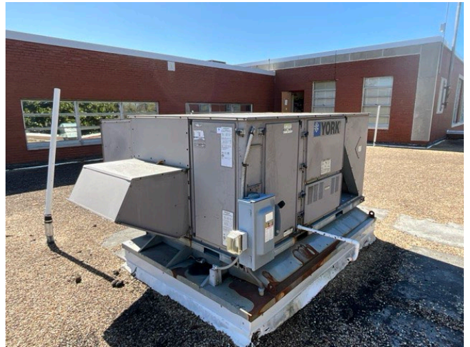
20 - HVAC, Roof top units
