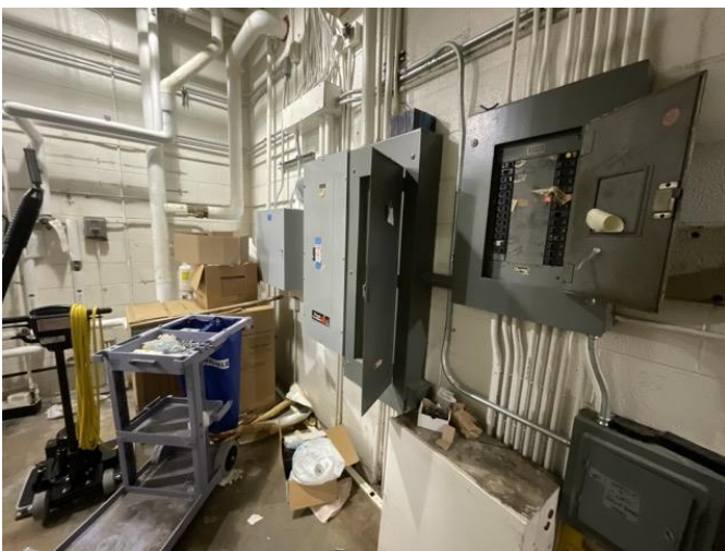
11 - MAIN ELECTRICAL DISTRIBUTION
