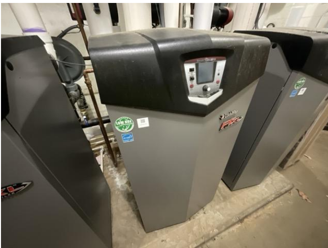
9 - MECHANICAL ROOM - HVAC BOILERS
