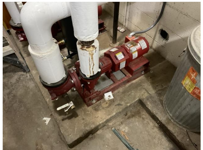
10 - HEATING WATER CIRCULATION PUMPS
