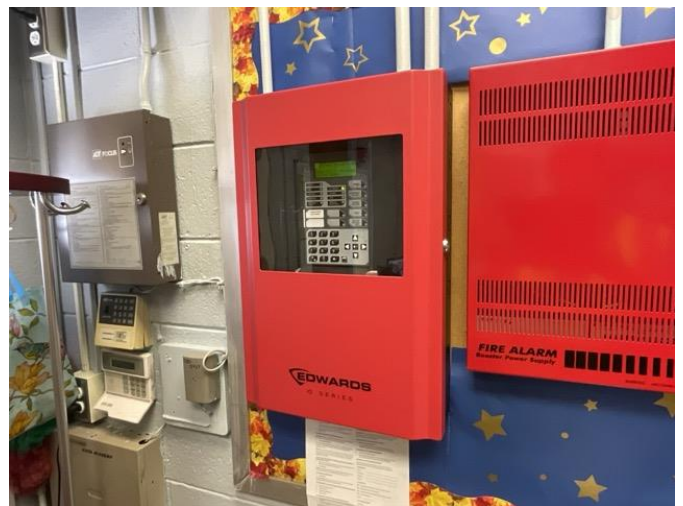
12 - FIRE ALARM PANEL
