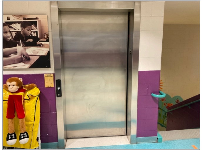
LOBBY LOOKING AT CAB
