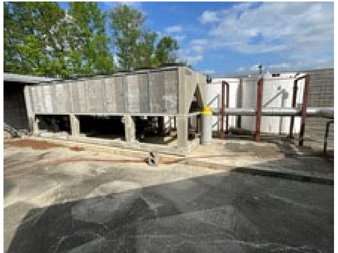
20 - CHILLERS AND PUMPS
