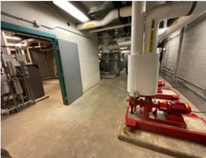
19 - SECONDARY MECHANICAL ROOM
