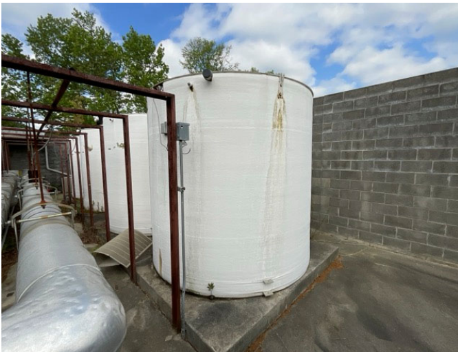
21 - WATER STORAGE TANKS
