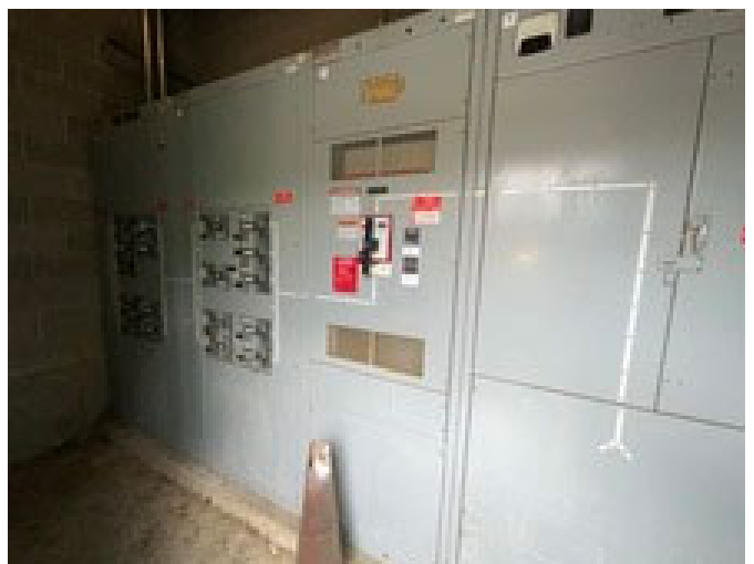
24 - MAIN ELECTRICAL SWITCHBOARD
