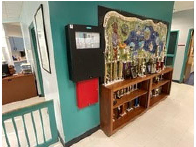
26 - FIRE ALARM PANEL
