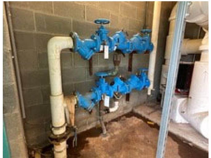
16 - DOMESTIC WATER PIPING
