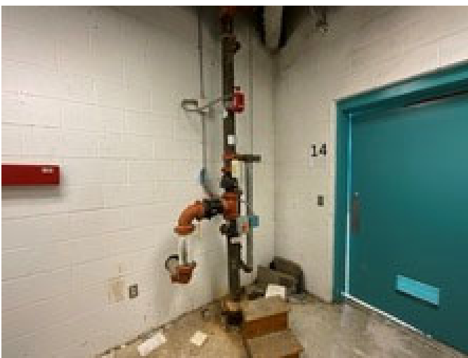
23 - FIRE SUPPRESSION SYSTEM
