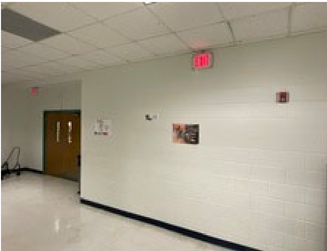
27 - FIRE ALARM DEVICES
