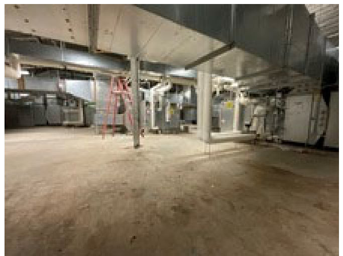
18 - MAIN MECHANICAL ROOM
