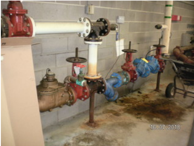
Domestic water service
