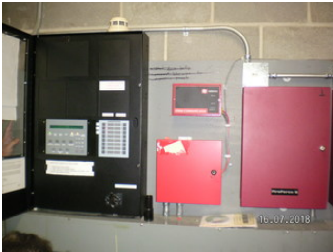
Fire alarm panel
