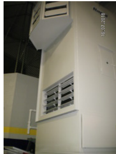
Direct fired unit
