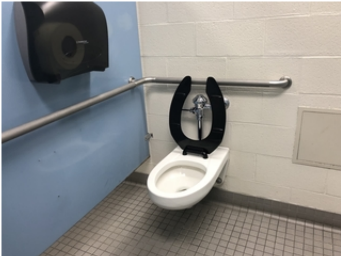
Non-Conforming Grab Bars
