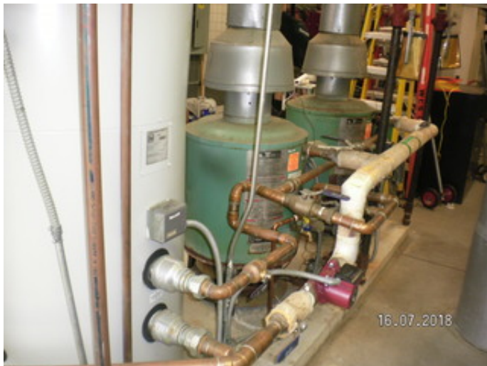
Original water heaters
