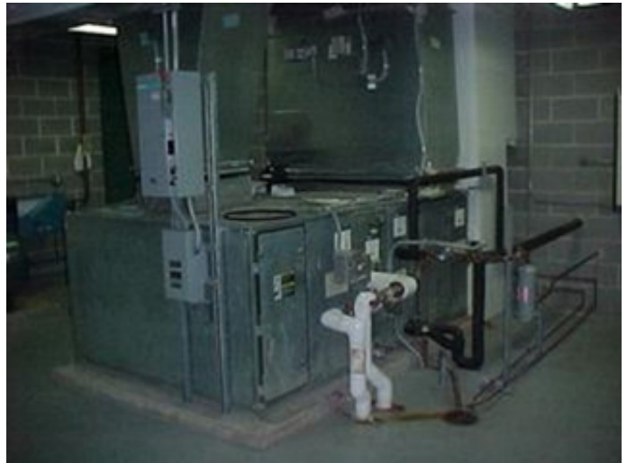
Air handling unit
