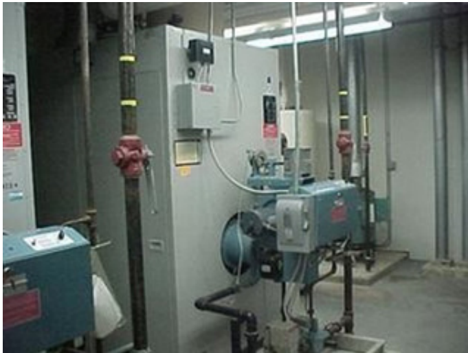
Hot water boilers
