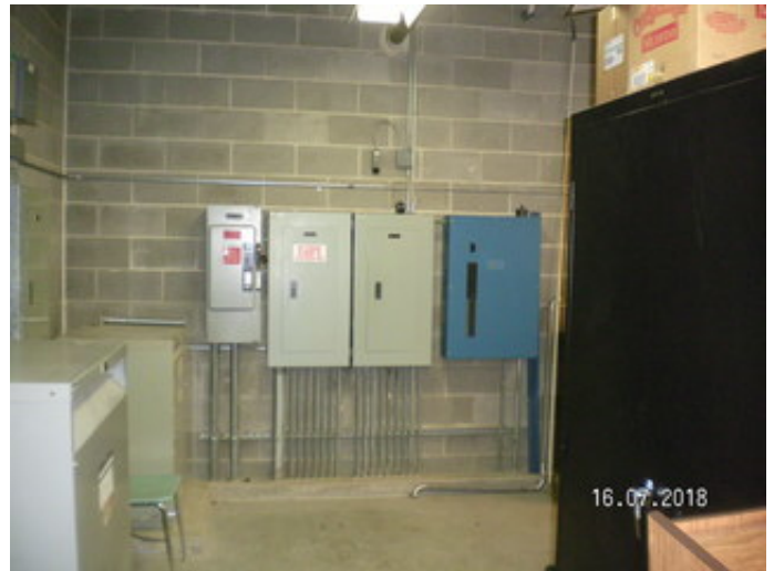
Electric room panels
