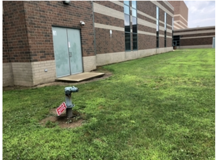
Fire department connection
