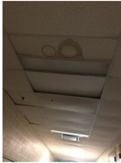
Damaged Acoustical Ceiling
