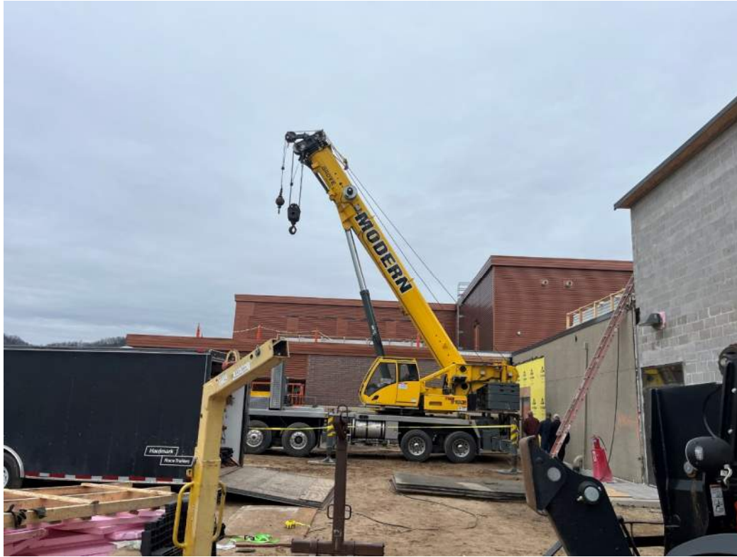
Solar Connection Solar Panel Install Began – Crane for Hoisting Material to Roof
