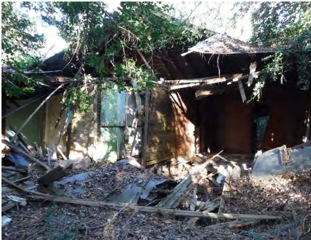
Photo 5: View of dilapidated house on the southern portion of the Site.
