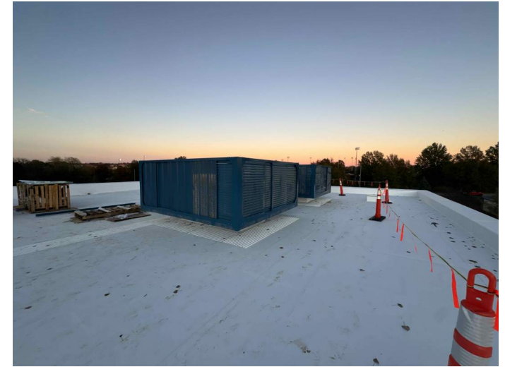
EPiC Elementary - RTU/Screens
