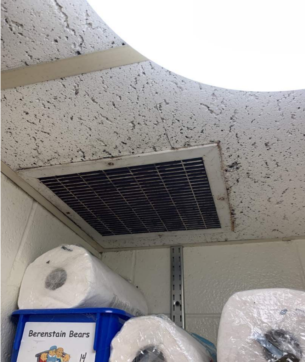
Room 18 - Bathroom Particulate accumulation/suspect fungal growth on ventilation diffuser
