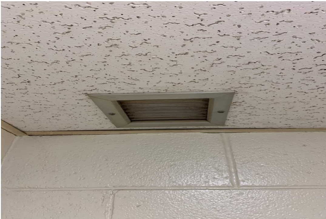
Room 19 Particulate accumulation on ventilation diffusers in classroom and bathroom
