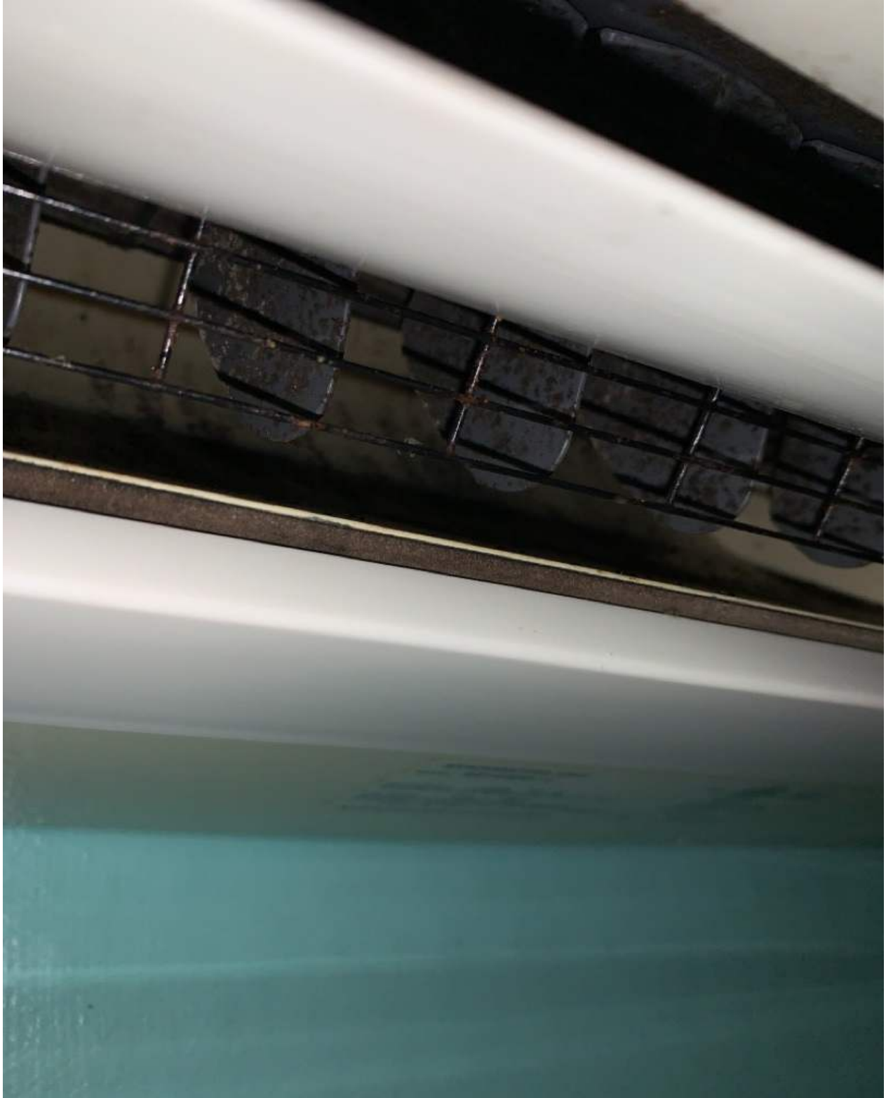
Room 18 – Wall -mounted ventilation unit displaying signs of particulate accumulation/suspect fungal growth within unit.
