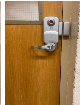
New Doors with Locks
