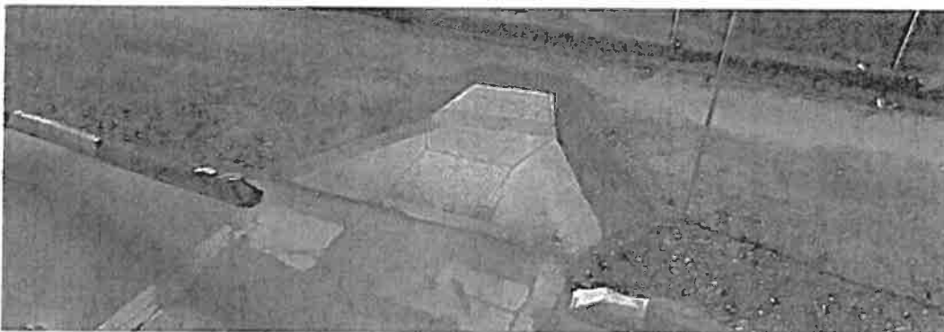
Photo 12: Ramp at School Crossing at Brookside Road, Stockton (Source: Google Street View)
