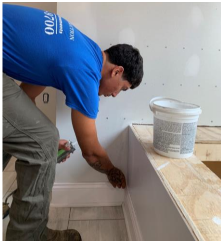
Co-op student Jesus Chavez (CH) helps the N&C Construction team at the end of the work day.
