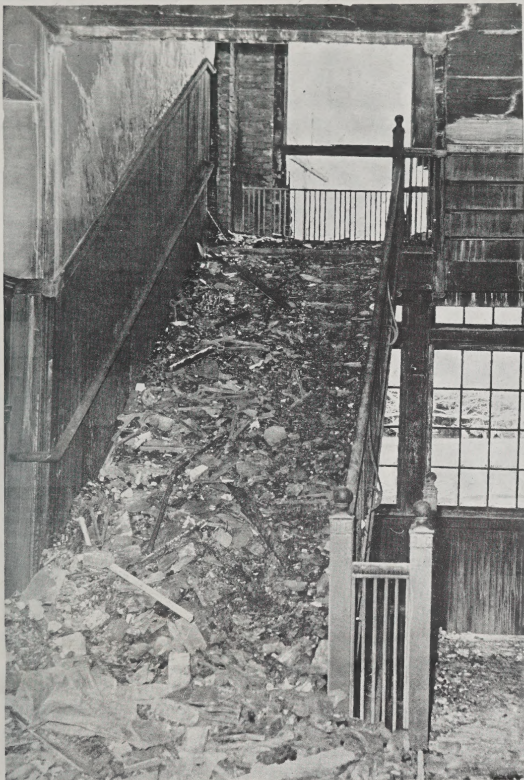
Once full of happy students, staircase outside Mr. Walter Bezubka's math room is covered with fallen debris, as reminders of what could have been a national disaster had the students been trapped in the inferno. (Photo by Stanley)
