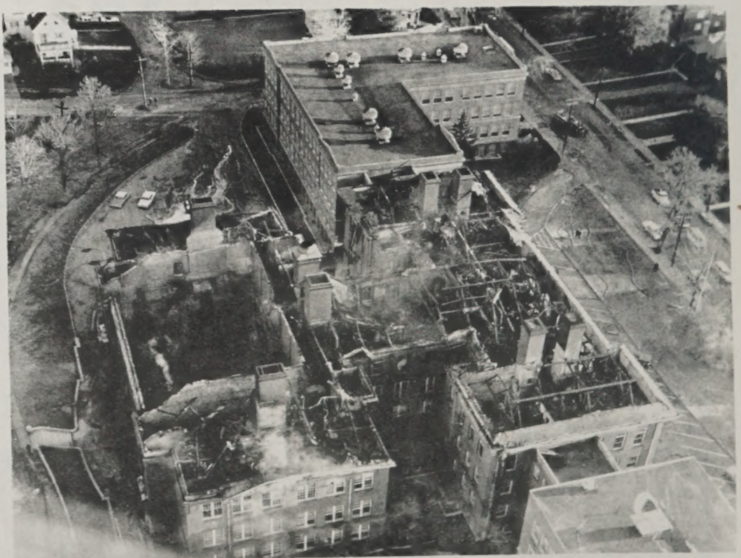
Boston Globe aerial shot captures burnt out remains of Buildings B and C.
