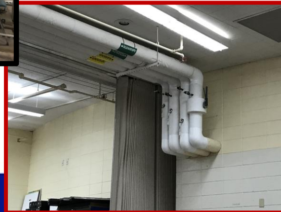
Winona ES – Hydronic Piping
