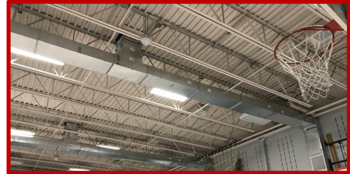
Ductwork – Various Locations
