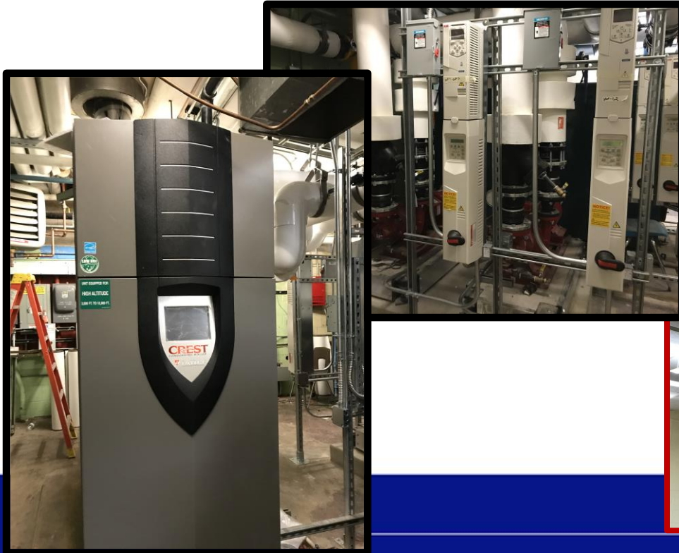
Berthoud ES – Boiler/Pumps
