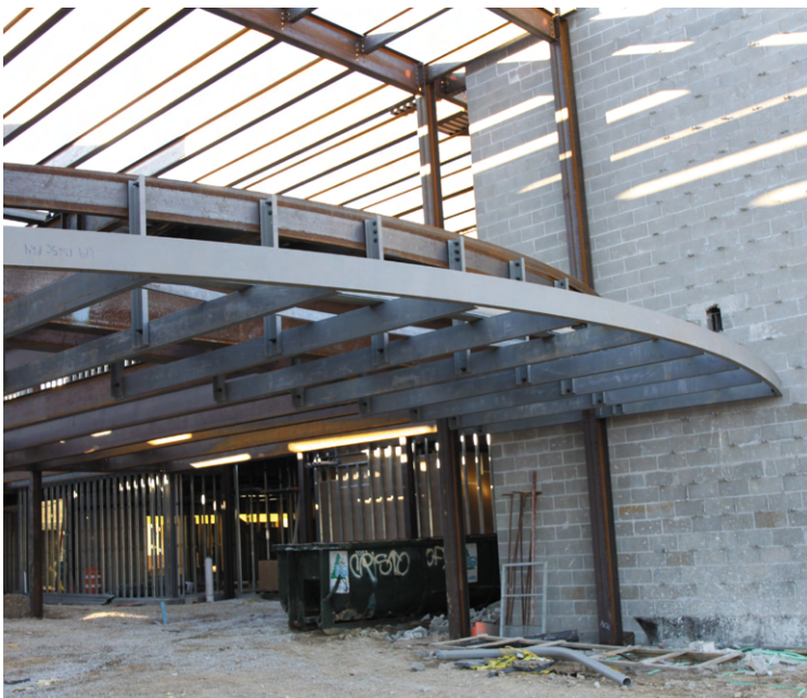
The Middle School entrance will lead to the 7th grade commons. Multiple commons areas throughout the school will provide ideal spaces for group meetings, studying and hanging out before and after school.
