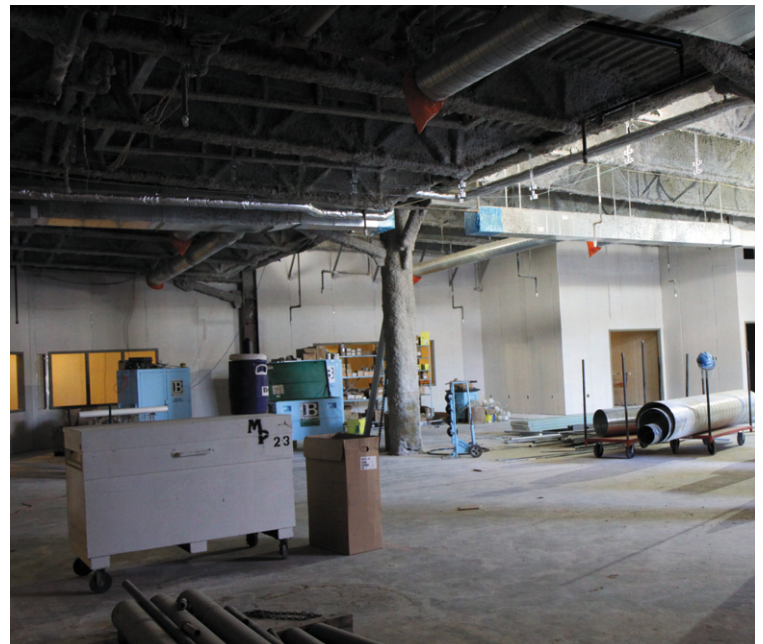
The expanded library at Town & Country will not only house many more books but will also provide storage for archives and spaces for students to collaborate and study.
