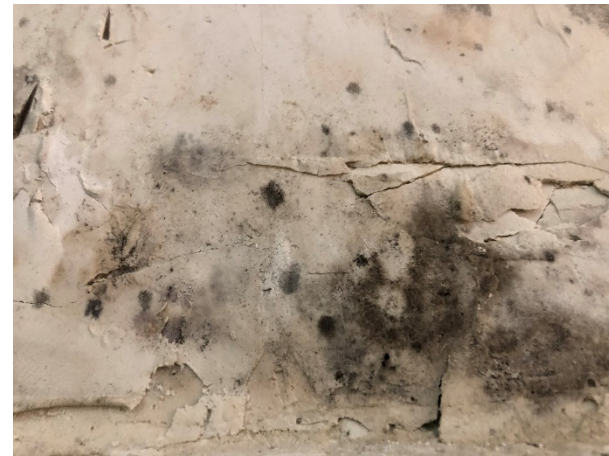
Francis C Hammond, Stairwell View of Mold
