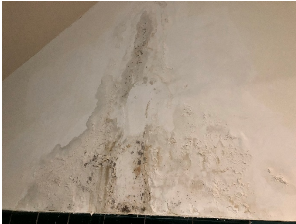
Francis C Hammond, Stairwell View of Water Damage
