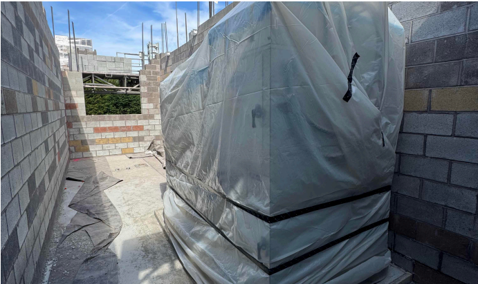
HVAC units in the mezzanine
