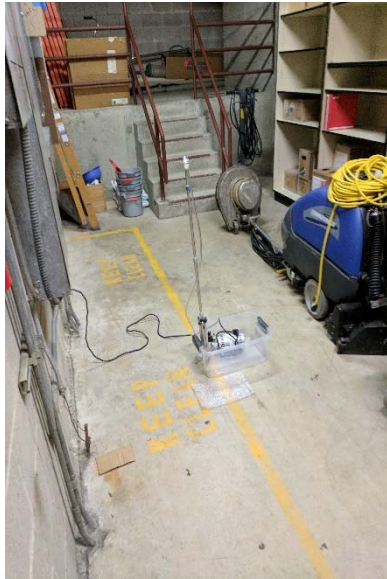
72517-GYM-Electric Room: small gymnasium electric room.
