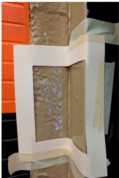
72417-GYM-Small Gym A: northwest door frame in small gymnasium.
