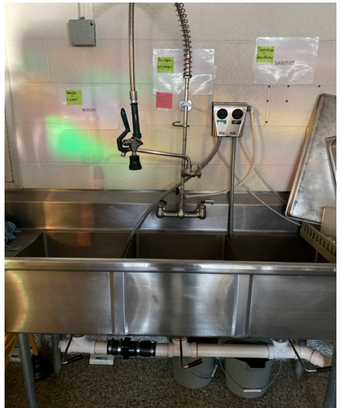
2/19/2024 - 8812-4 - Three Trails - Kitchen-Southwest Sink
