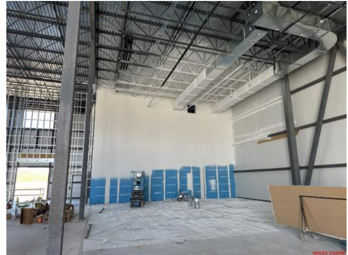
Dryfall Above Freezer
