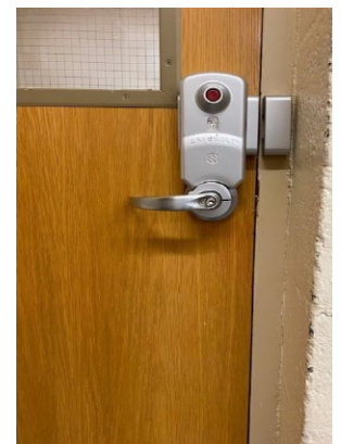
New Doors with Locks
