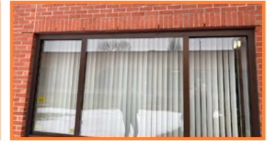
Windows in Need of Replacement
