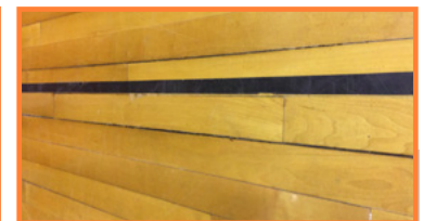
Worn Gym Floor at Jr./Sr. High School
