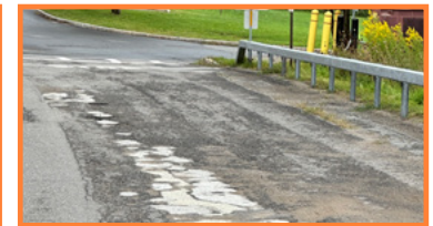
Erosion of Asphalt Drives Across Campus
