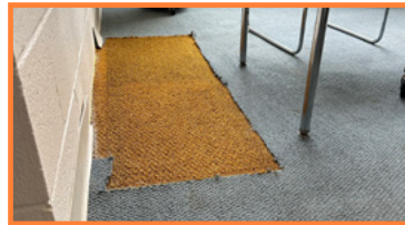
Carpet and VCT Flooring in Need of Replacement at Elementary School
