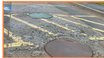
Deteriorating Concrete Pad at Elementary Fuel tank
