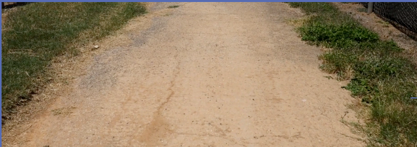
SOFTBALL WALKWAY NOT ADA ACCESSIBLE
