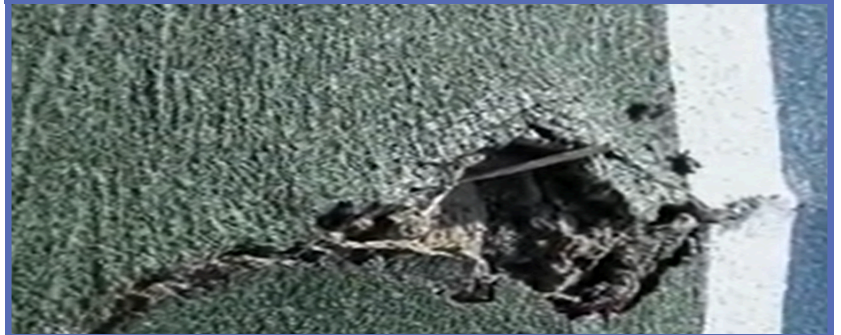
CRACKS IN COURTS
