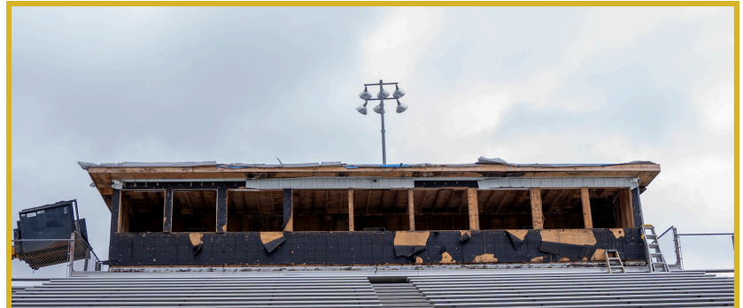
PRESS BOX WAS CONDEMNED AND REMOVED
