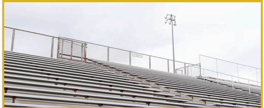
BLEACHERS HAVE NOT BEEN UPDATED SINCE 1982, SHOWING ADA ACCESSIBILITY ISSUES
